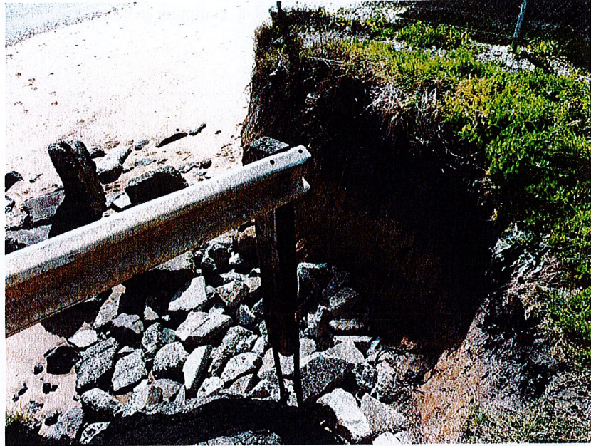
Photo 2. Western view of coastal bluff edge and broken concrete (2/22/2018).
