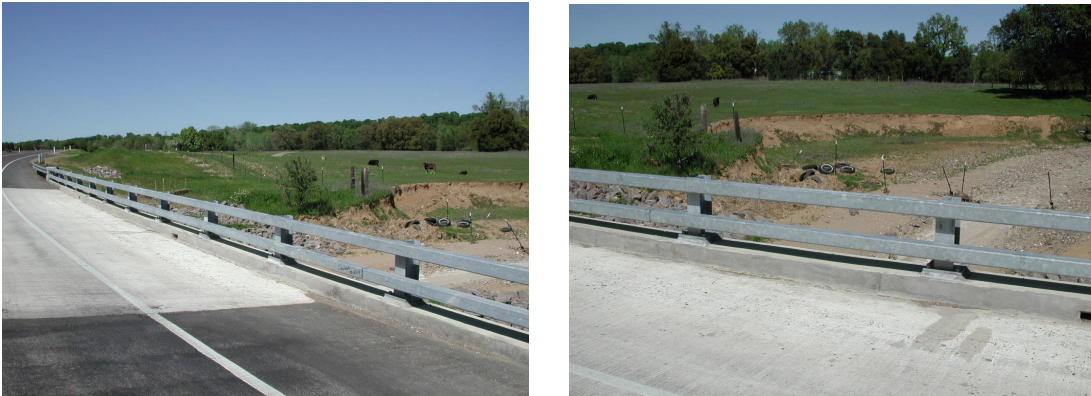
Figure 3.4.1c Alaska Bridge Railing (Note: Barriers shown here do not include the pedestrian/bicyclist railing that is required for this project)
