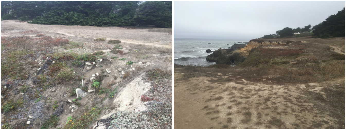
Figure 3 Photos of the bluff top showing concrete debris and fill at the top of an active landslide (left) and the variability in the bluff edge caused by gullies (right)
