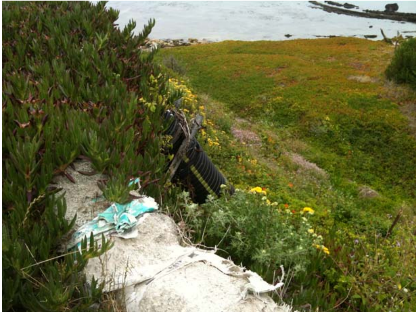
A retaining wall of degraded plastic sandbags at Ellendale in Moss Beach – Sunshine Valley watershed outlet to Fitzgerald Marine Reserve
