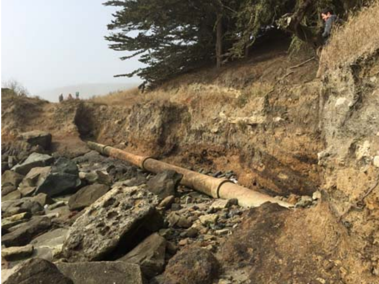
Exposed 14" OD abandoned sewer pipe containing asbestos presents construction challenges.
