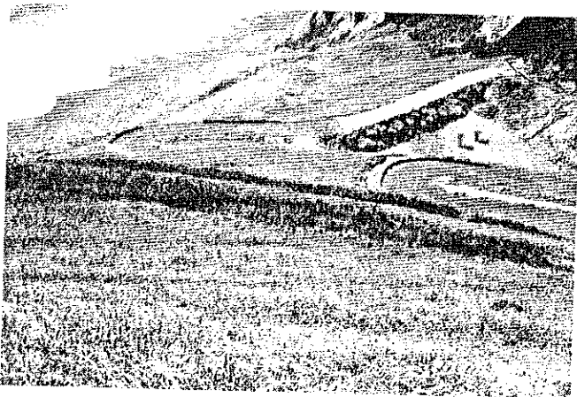
Avalon Canyon Slide Repair - March 1999 - Quick Cover
