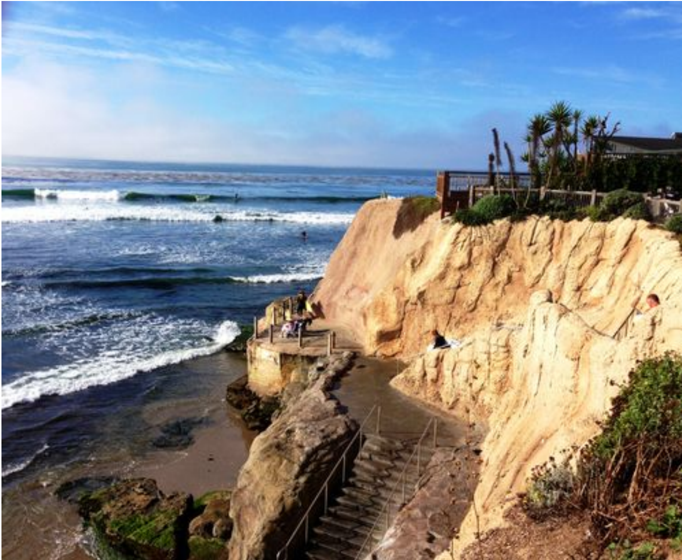
Contoured concrete tie-back seawall with beach access stairs Pleasure Point, Santa Cruz, 2011
