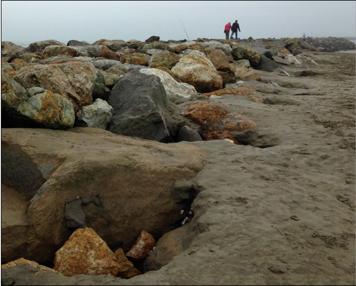
Figure 49. Photograph showing areas of scour due to surging along the harbor side of the east breakwater (Source: James Zoulas)
