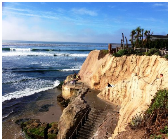
Contoured concrete tie-back seawall with beach access stairs mimics the natural cliff face. (Pleasure Point, Santa Cruz)
