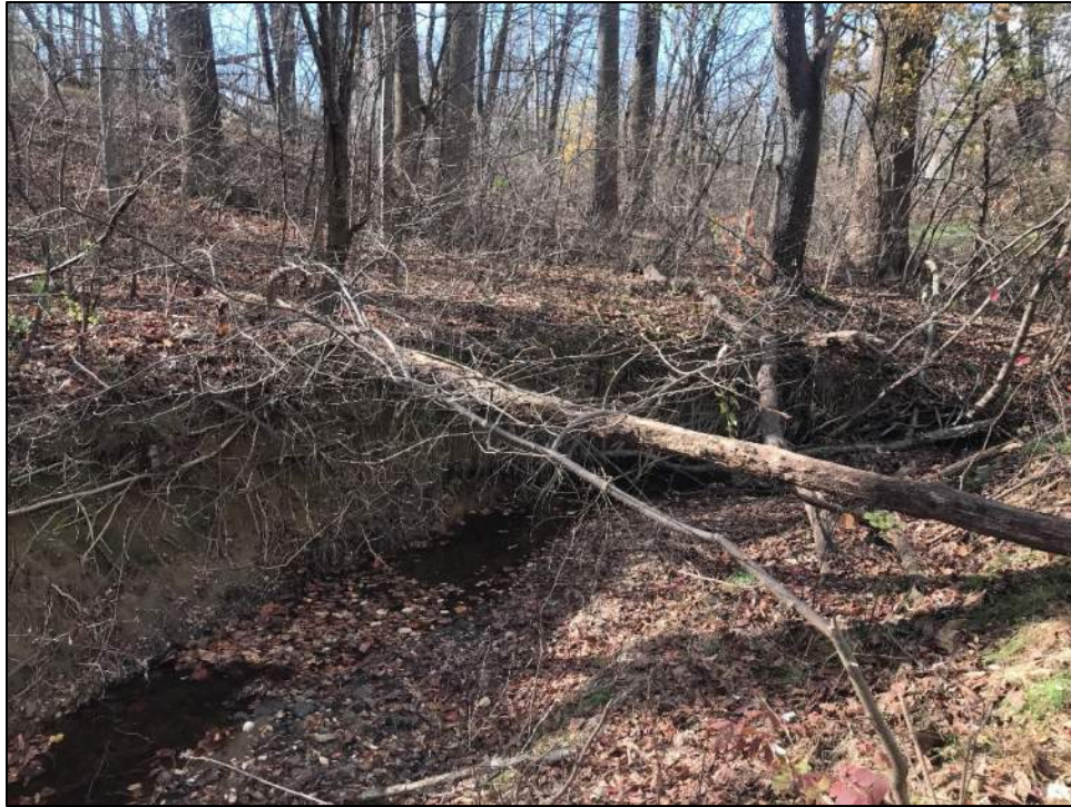
Photo 7: Reach 4, looking downstream towards Reach 3A, 3' actively eroding bank.
