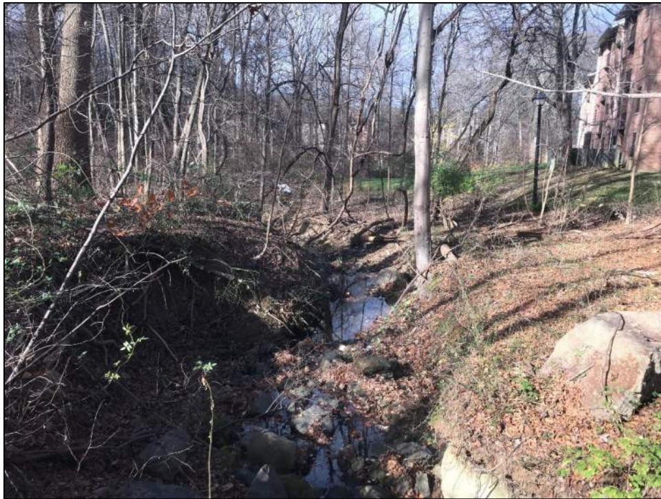
Photo 10: Reach 7, looking downstream near Cloudleap Ct, 3' actively eroding bank with minimal riparian vegetation.
