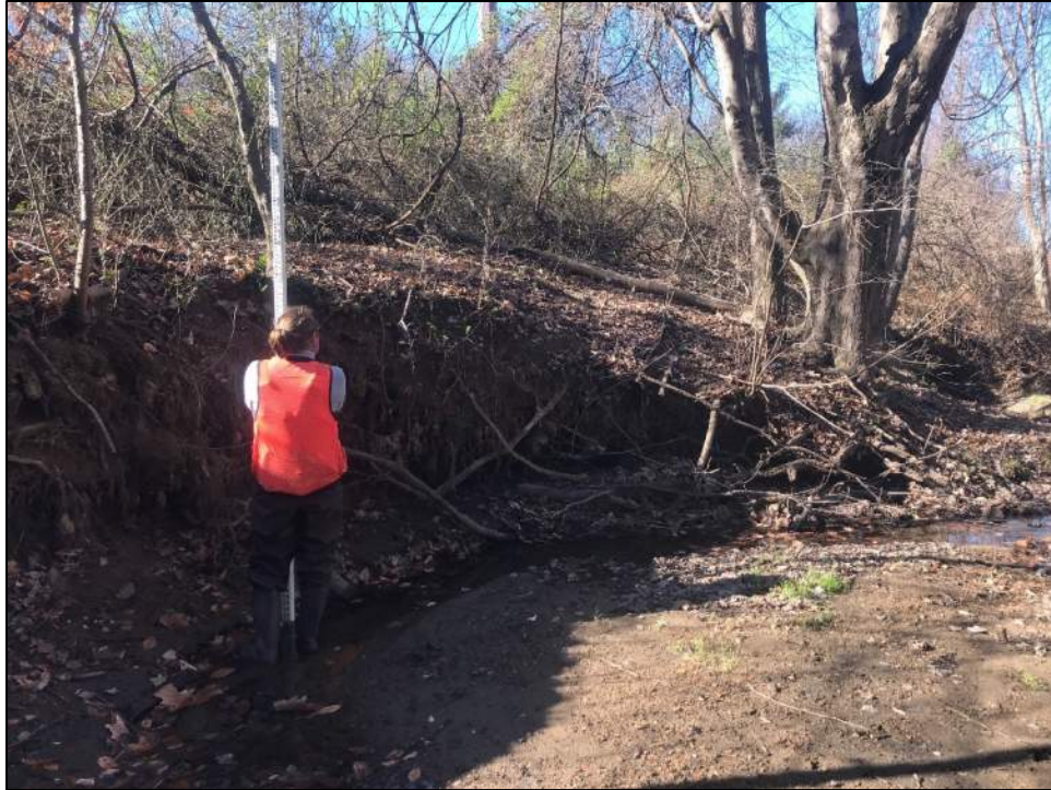
Photo 31: Reach 23, looking upstream near Hourglass Place, 6' eroding banks.
