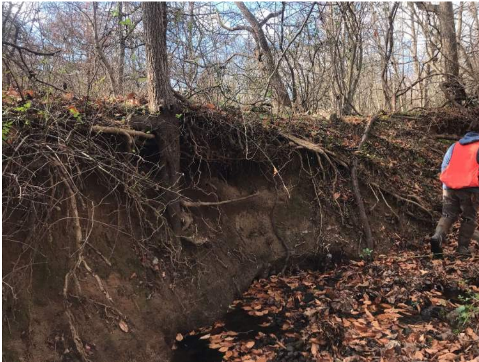
Photo 4: Reach 3-1, looking downstream towards Reach 3A, 4' actively eroding stream bank.
