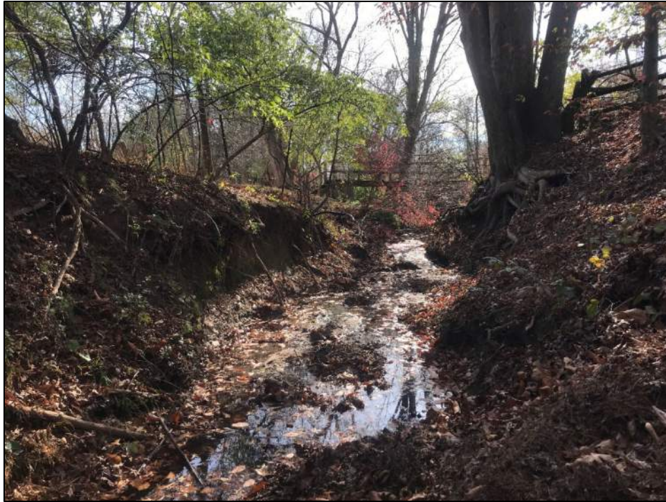
Photo 19: Reach 14, looking downstream near Tamar Drive, 4' actively eroding bank. The riparian area contains a high concentration of invasive species.
