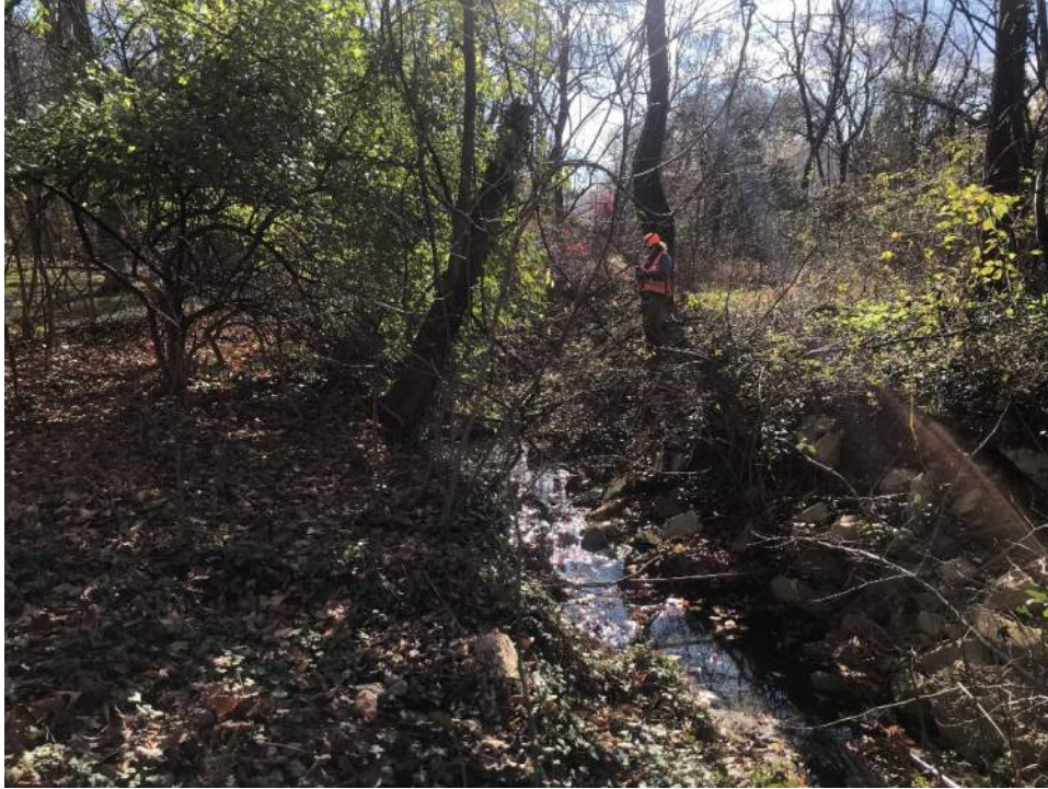
Photo 3: Reach 2, looking downstream near Blade Green Ln, 3' actively eroding stream banks. The riparian area contains a high concentration of invasive species.
