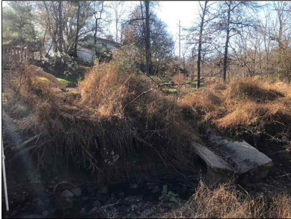
Photo 29: Reach 21A, looking at concrete swale near DeerPasture Dr, swale is disconnected from the stream and near failure.
