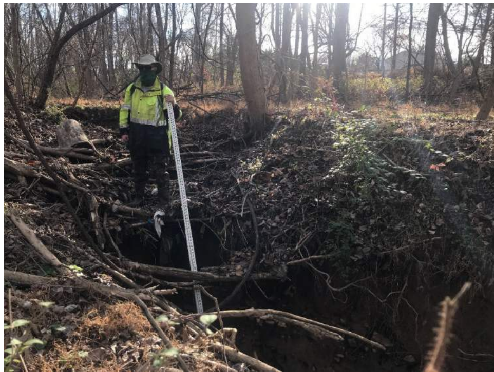
Photo 28: Reach 20, looking upstream near Oakland Mills Rd, 9' head cut and actively eroding banks.
