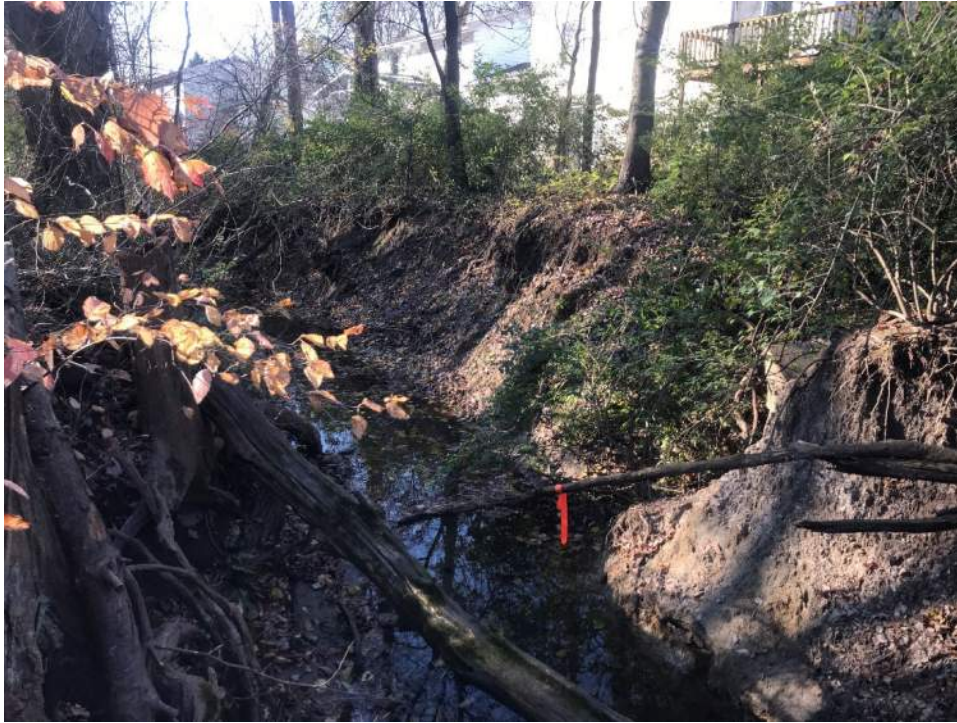
Photo 1: Reach 1A, looking downstream, 4' actively eroding stream bank.
