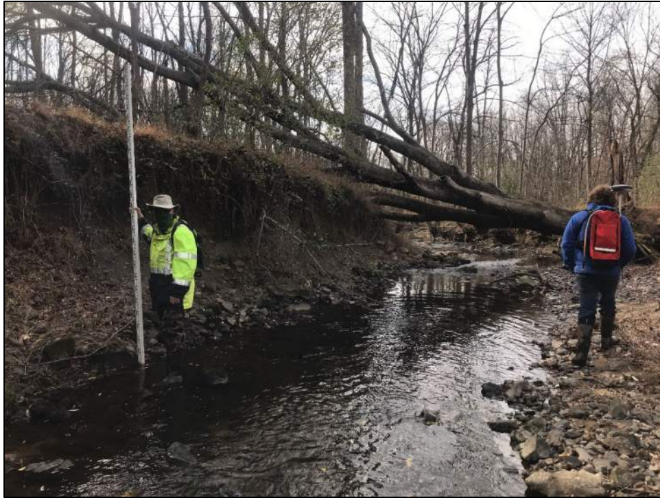
Photo 21: Reach 15A, looking downstream near confluence with Reach 16, 8' actively eroding bank and large fallen tree.
