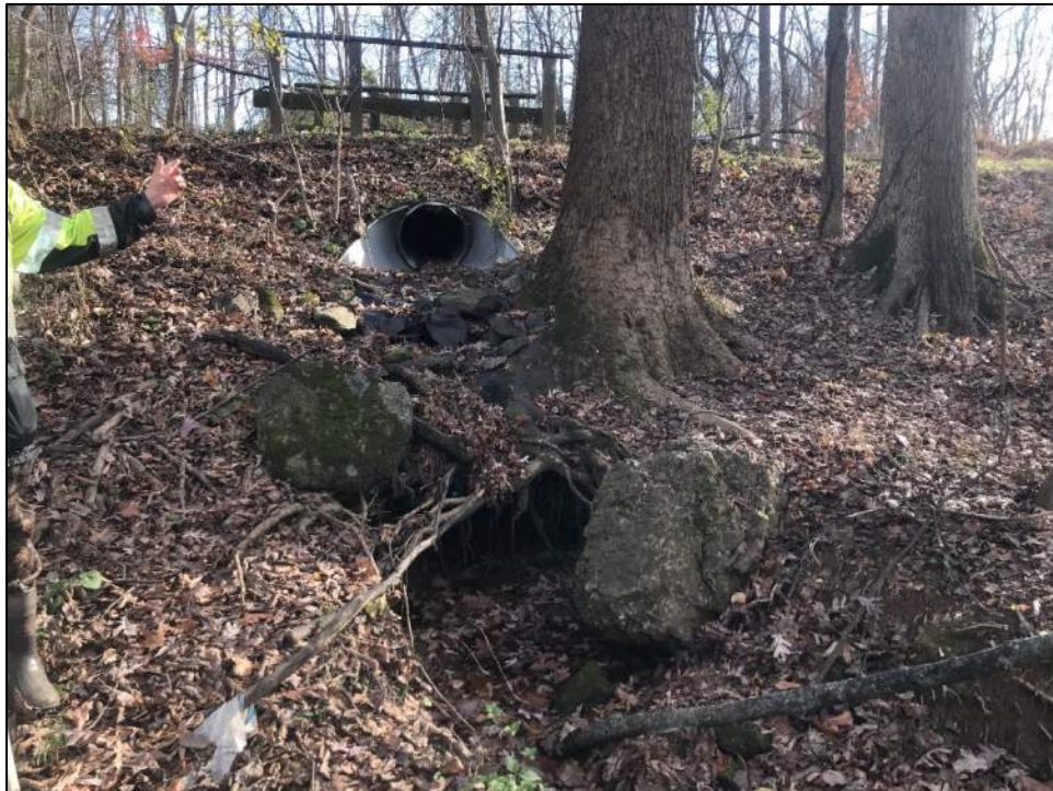
Photo 20: Reach 15-2, looking upstream near culvert under a pedestrian path, 2' head cut that is beginning to undercut a tree.
