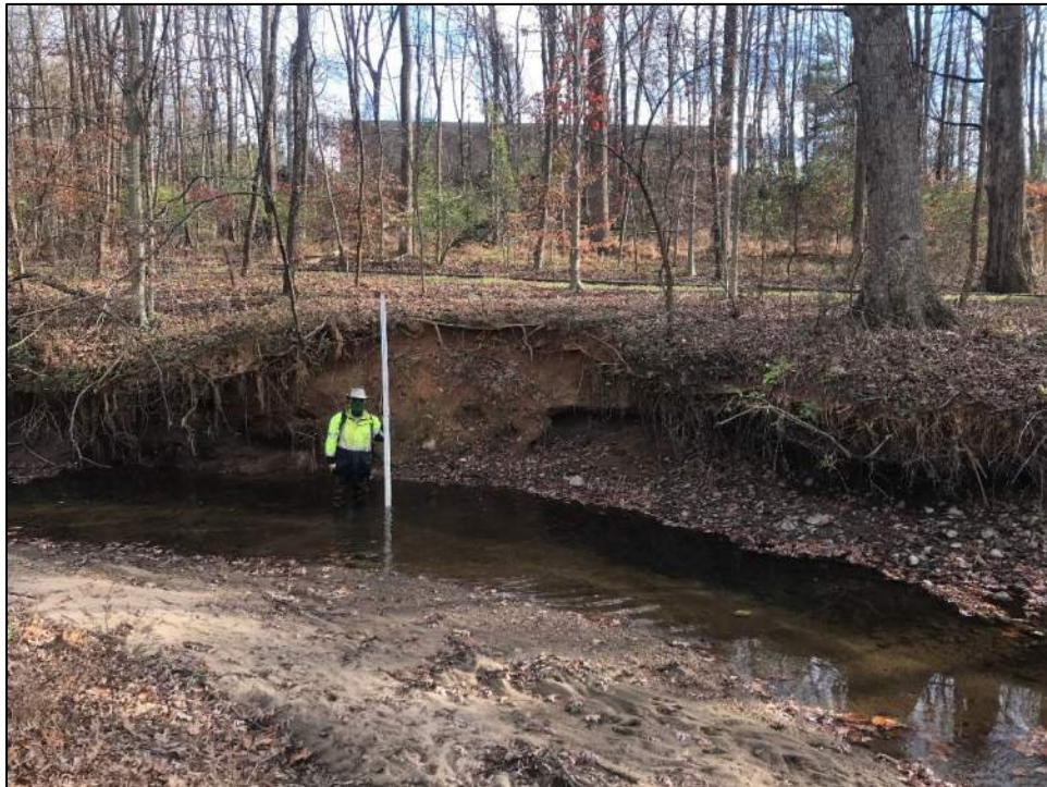
Photo 22: Reach 15B, looking upstream near Oakland Mills Rd, 9' actively eroding bank undercutting large tree
