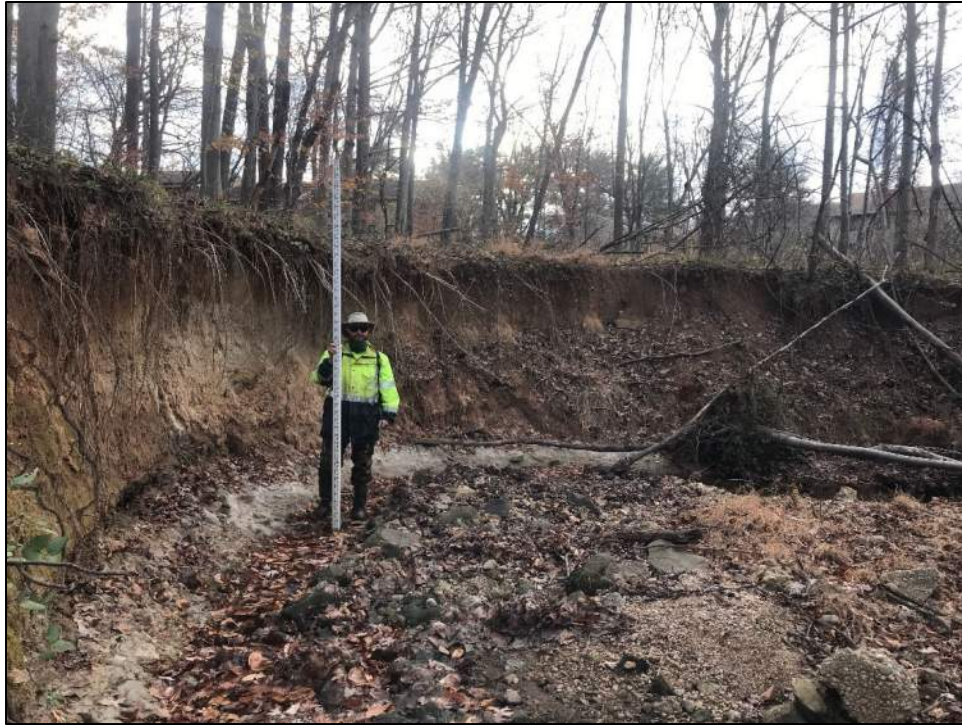
Photo 9: Reach 6, looking downstream near Tamar Drive, 9' eroding bank.
