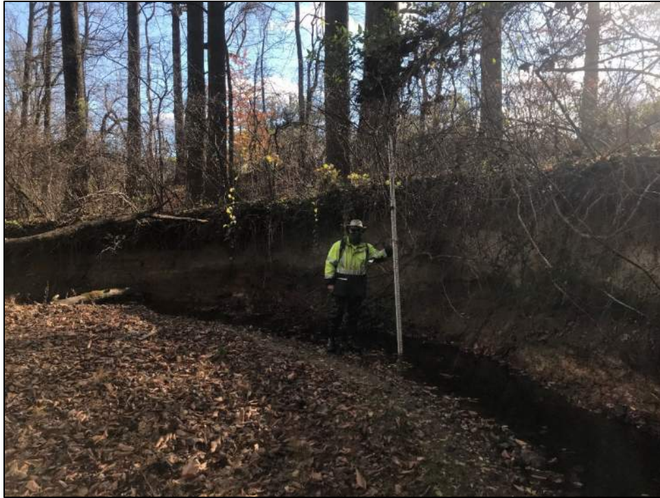
Photo 5: Reach 3A, looking downstream towards Lamb Skin Ln, 6' actively eroding bank.
