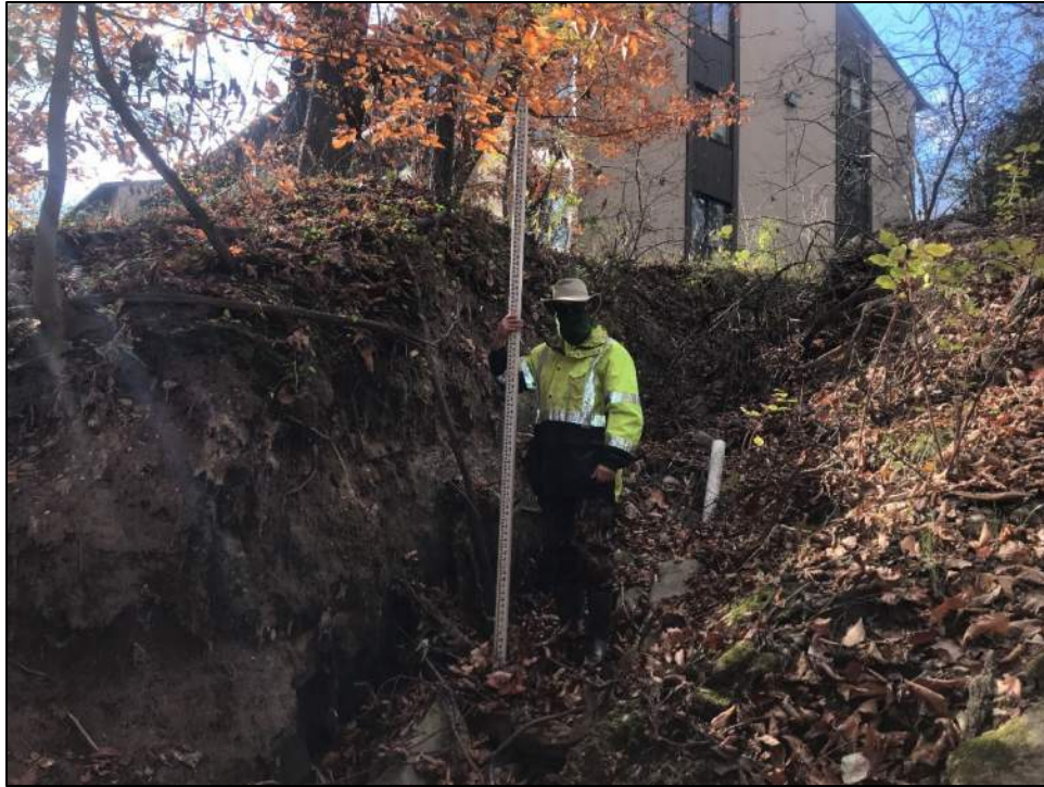
Photo 15: Reach 10, looking at side channel near the corner of Tamar Drive and Route 175, 7' eroding bank where apartment complex outfall meets Reach 10.
