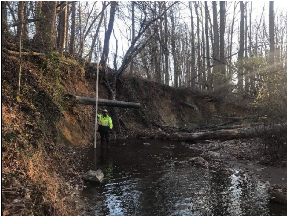
Photo 12: Reach 8B, looking downstream near Route 175, 12' actively eroding bank with disconnected and exposed pipes.
