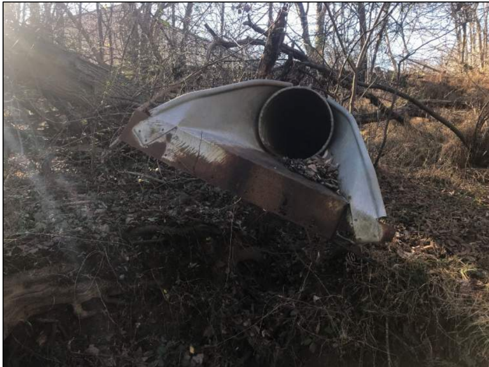
Photo 26: Reach 17, looking at outfall near Dobin Rd, the pipe has broken and is disconnected from the reach.
