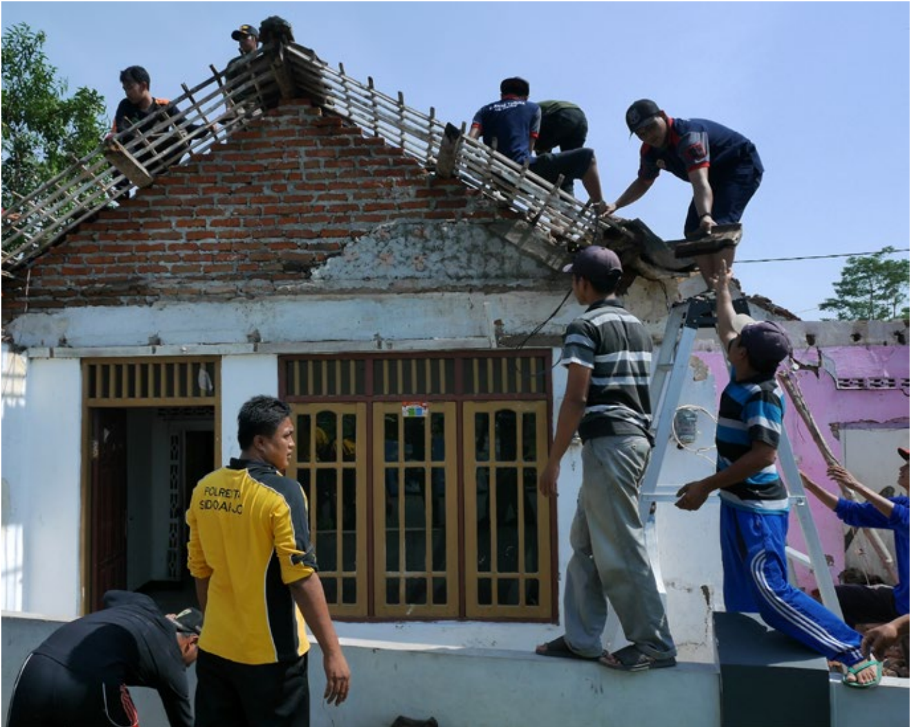
The people of Tulangan village work together to rebuild the houses of residents that were damaged by the tornado in 2018, East Java province, Indonesia. Photo: Shutterstock.
