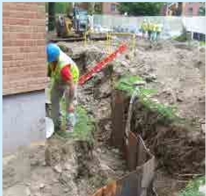
Passive impermeable barriers below grade stop water infiltration and protect building foundations. The left and center photos show vertical sheet piling being installed at Baruch Houses in Manhattan. The right photo shows flexible liners being installed below grade at Wald Houses in Manhattan (Credit: NYCHA)
