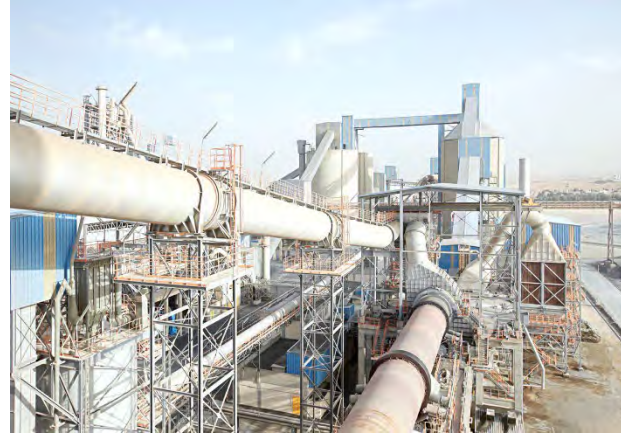
(Photo: ABB Cement)
