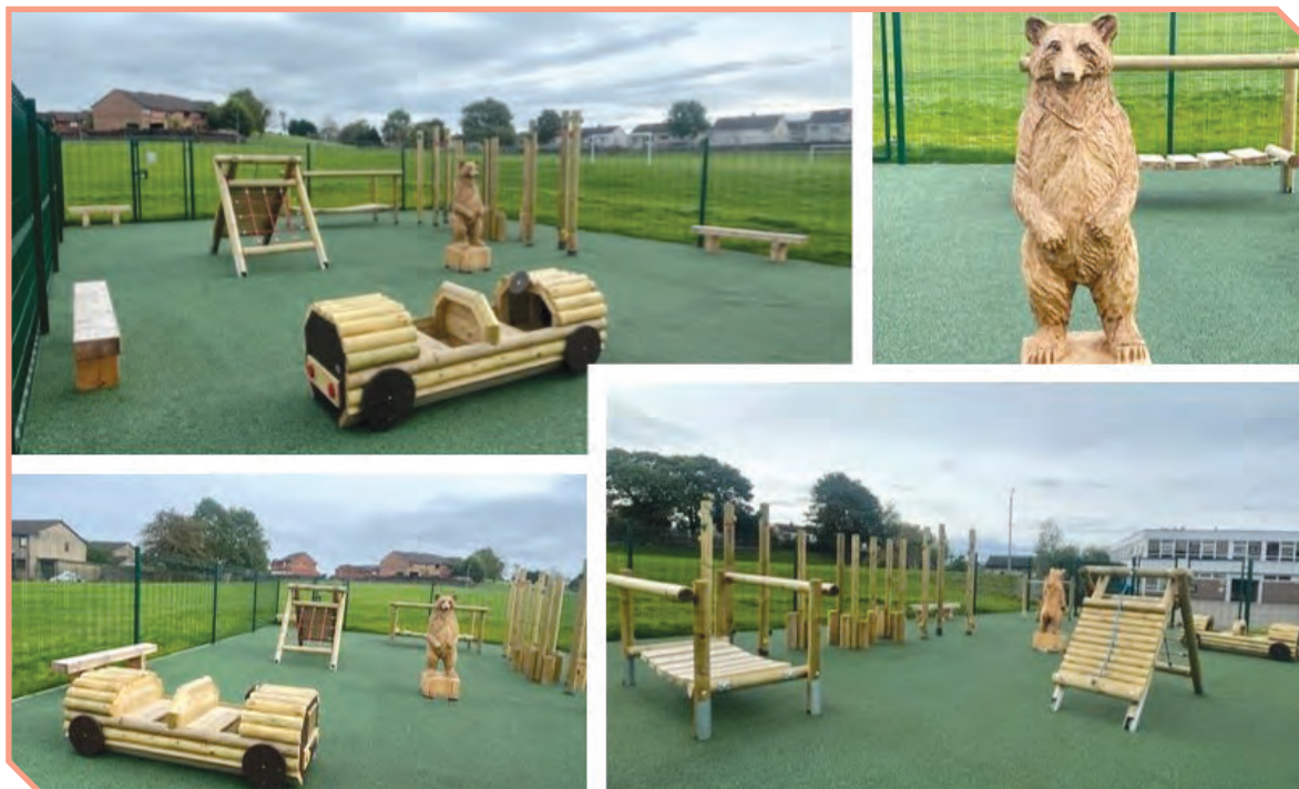
'The Cubby', the new play area complete with wet pour surfacing and play equipment.
