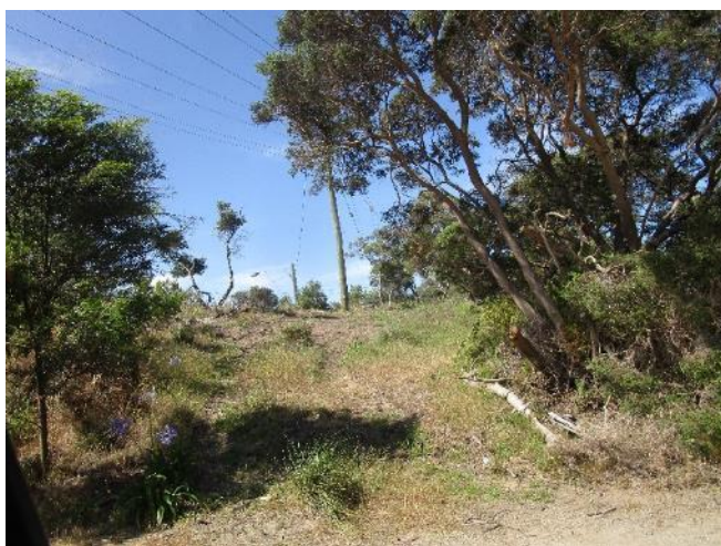
Vegetation and woody weed removal for power pole installataion - corner of St Johns Wood Road
