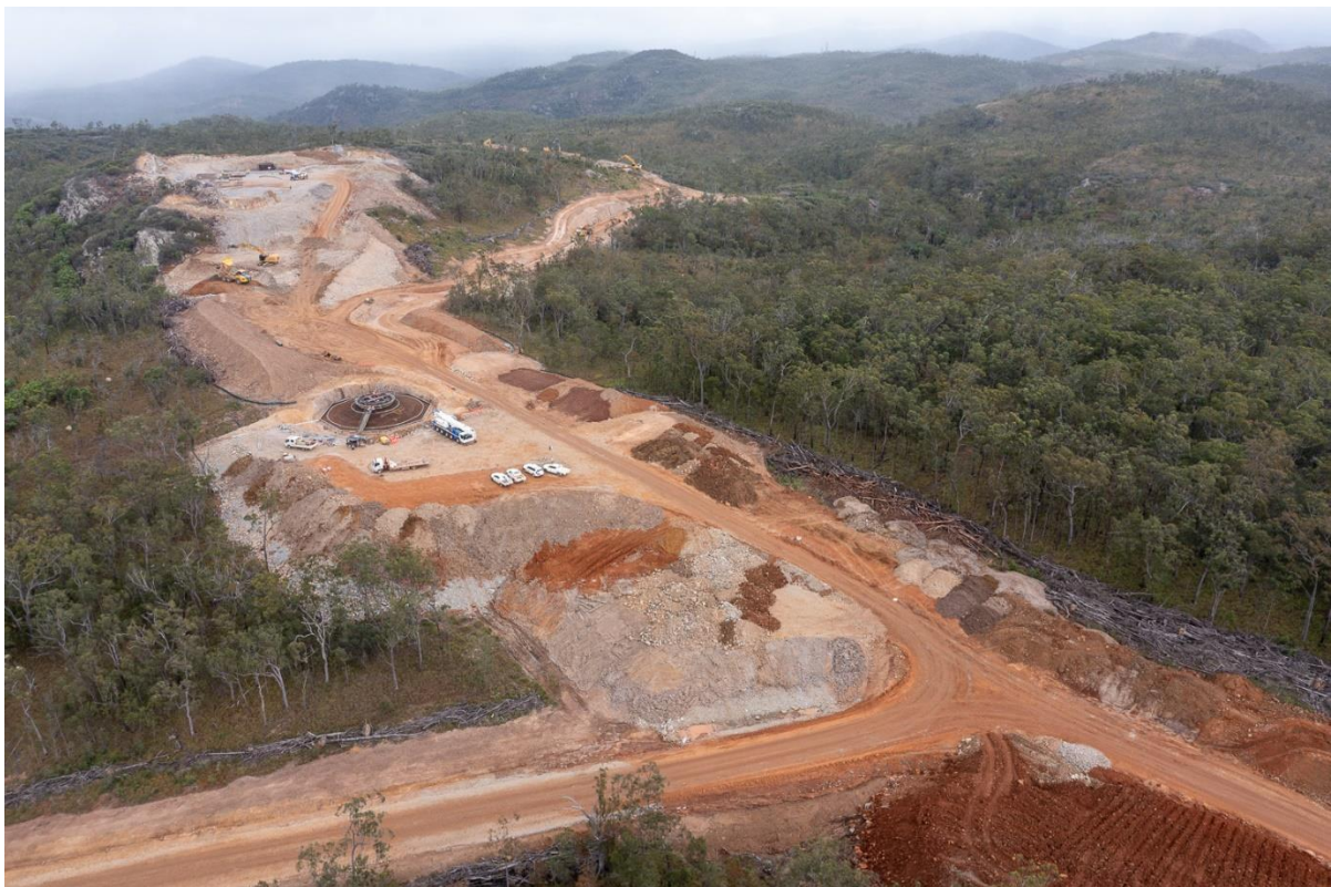
Figure 2. Very small section of the Kaban windfarm (under construction). Photo Steven Nowakowski.
