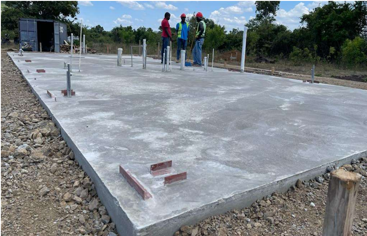
Photo 1: The slab foundations cured for roughly 10 days prior to beginning timber assembly.
