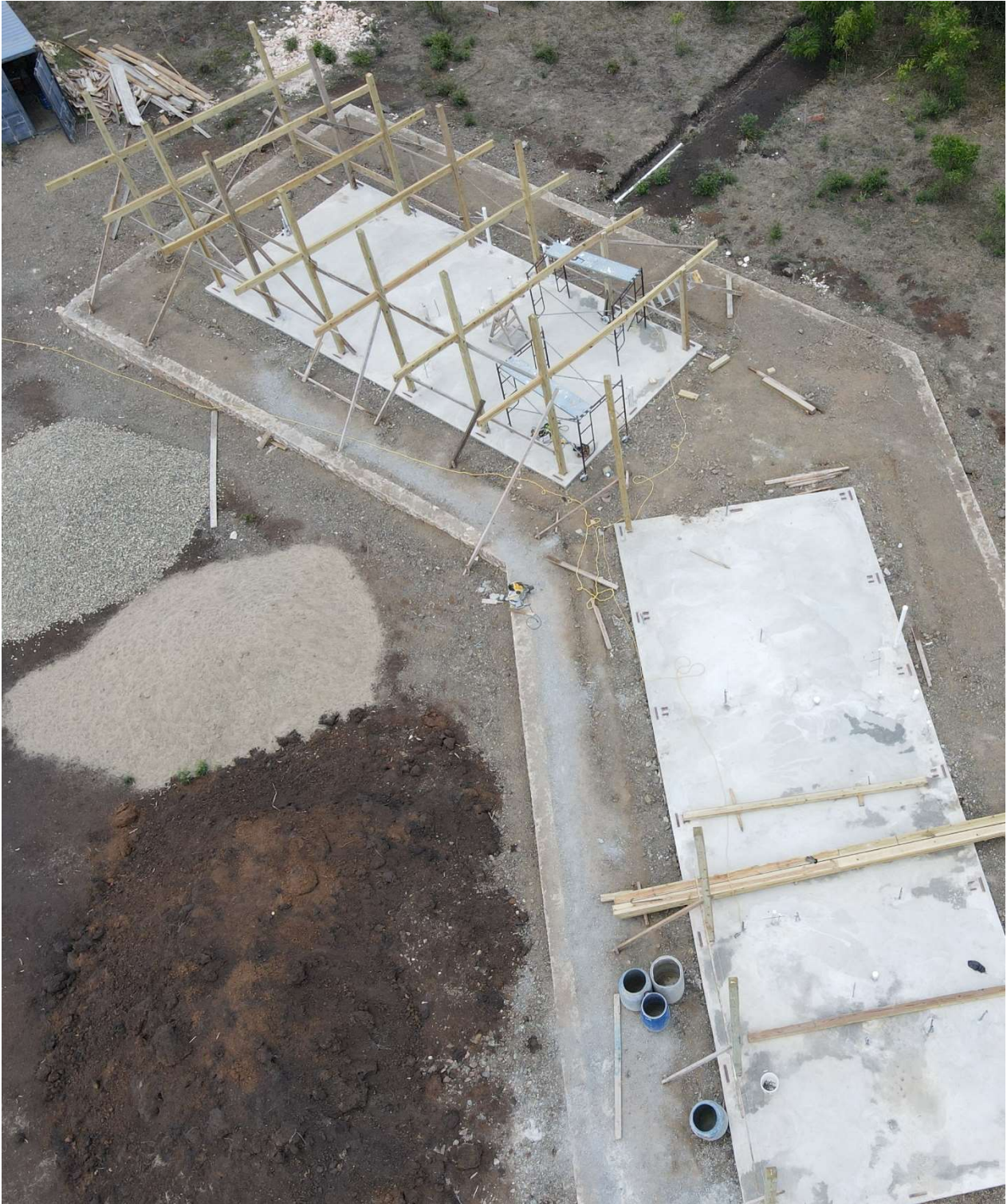
Photo 4: Rafters fixed prior to cutting column flush to rafter. Temporary braces were added and will be removed as the Rammed Earth Wall is formed up.
