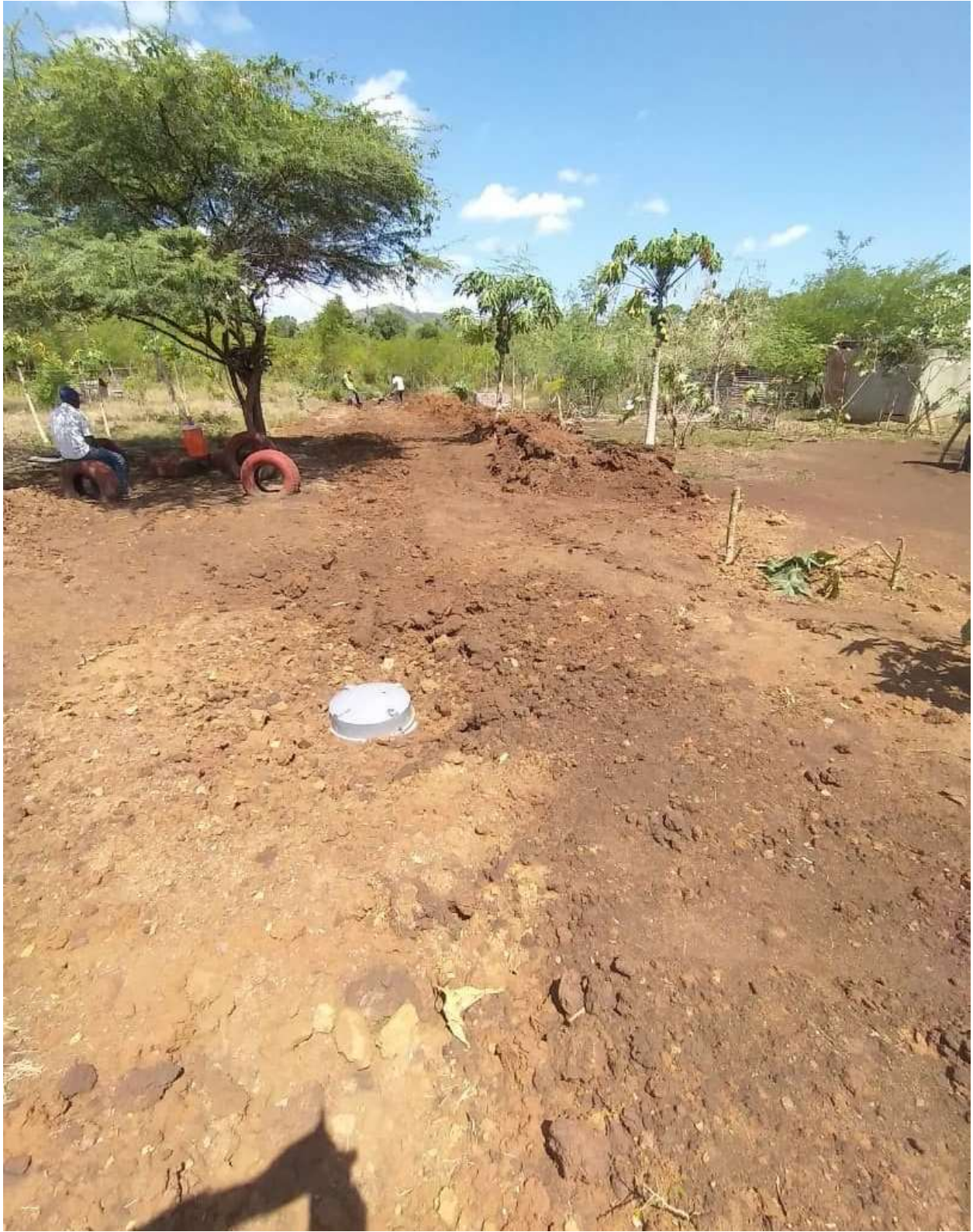
Photo 3: Septic tank and leaching line were installed, and the impacted areas are regraded.
