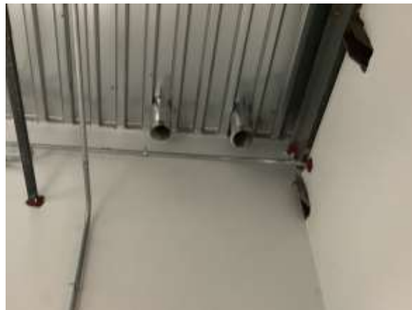
Figures 10 and 11: Examples of how conduit has been pre-installed to ensure the building is PV-ready.
