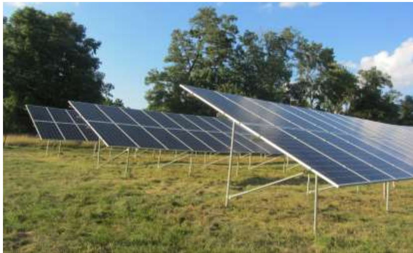
Figure 5: An example of a screw driven ground mounted PV system.
