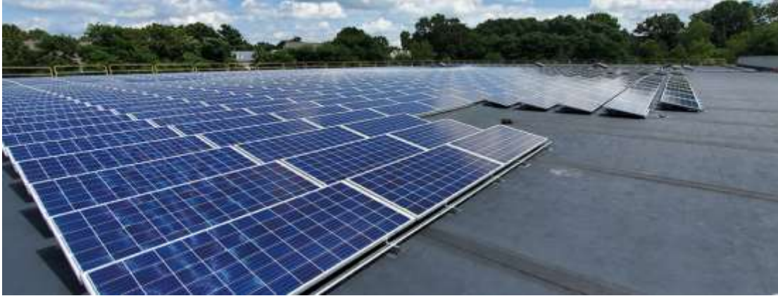
Figure 8: An example of a PanelClaw clawFR roof mounted ballasted PV system.
