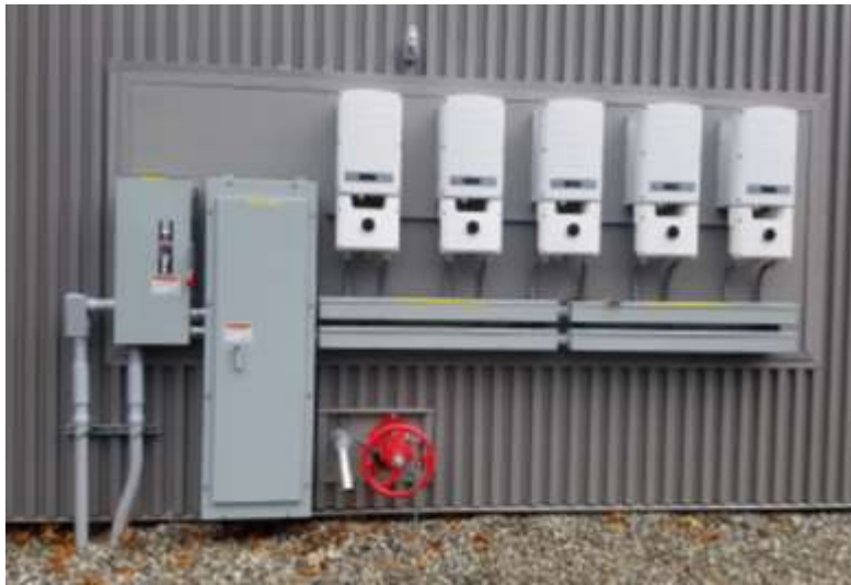
Figure 9: An example installation of PV inverters with a PV combining panelboard and AC disconnect switch.
