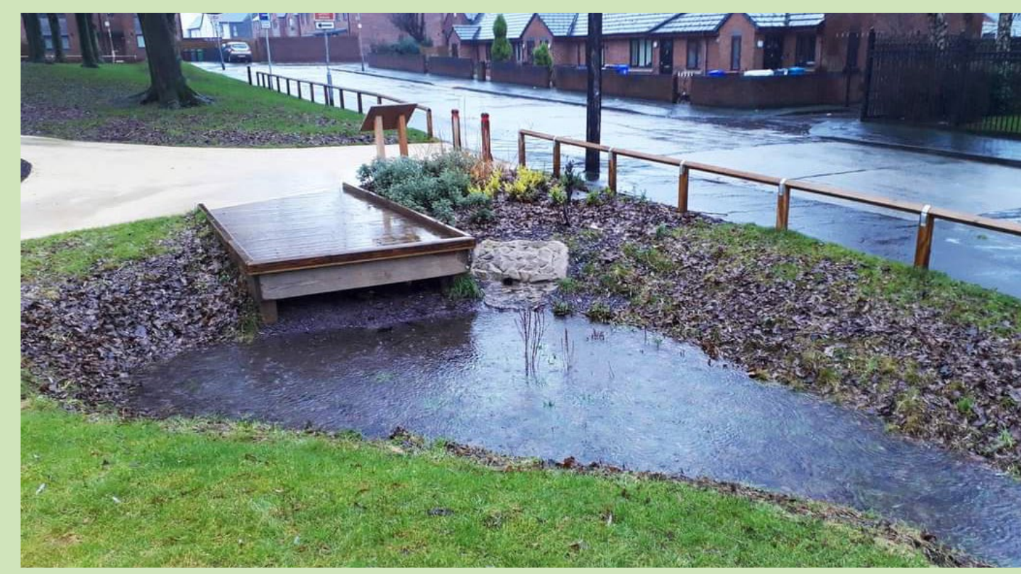
Swale filled with rainwater during Storm Christoph 2021 (James Rothwell)
