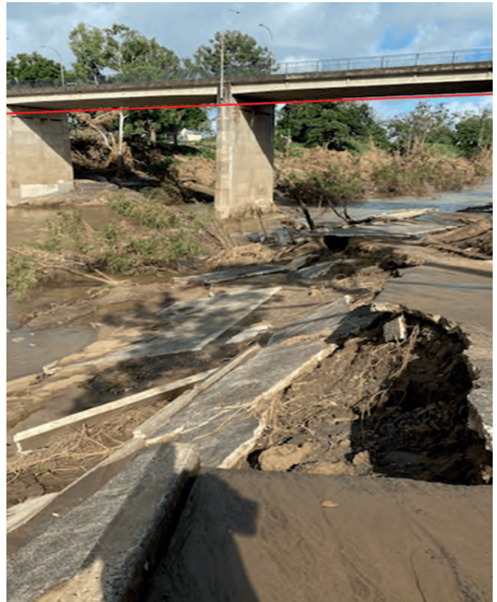
Figure 3: The Richmond River in Casino beneath the Irving Bridge. Red line indicates the approximate peak height of flooding on the 27th of February. Note the destroyed roadway and trees lain over by the force of flood water. (Photos courtesy of Risk Frontiers 2022)
