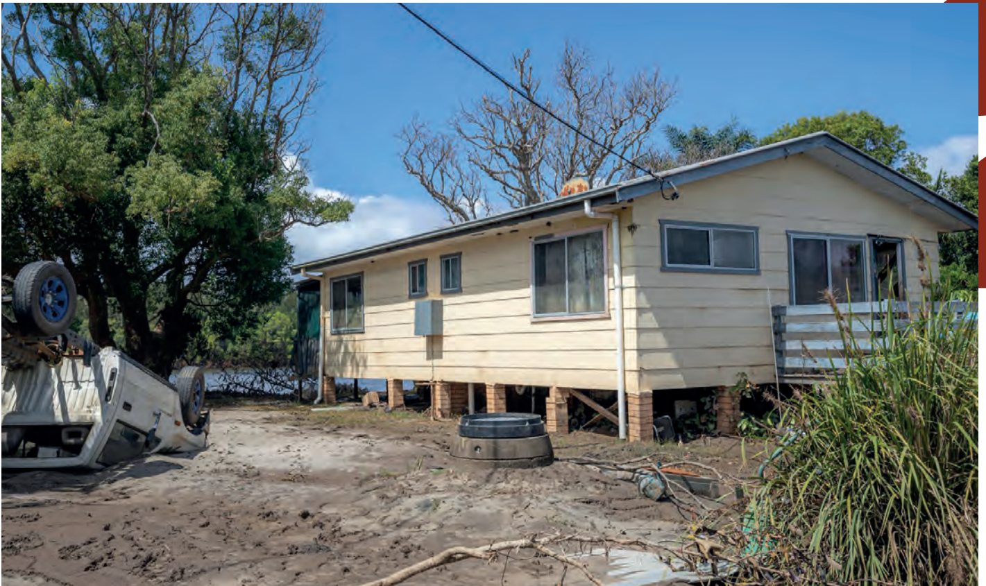
©Kristopher Cook Photography (c) 2022 Bundjalung Man One of the many homes destroyed on Cabbage Tree Island
