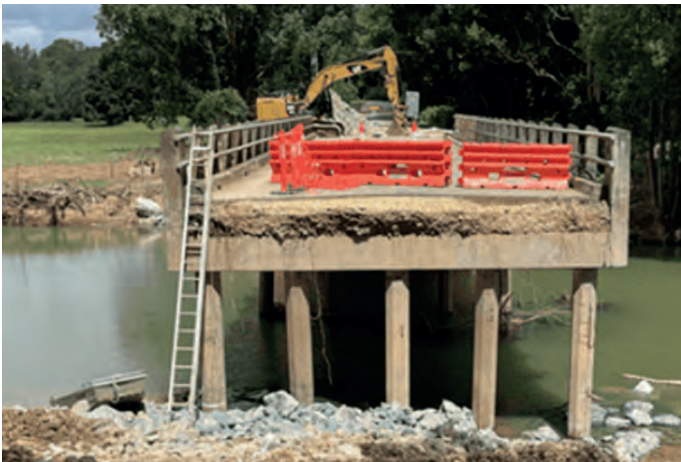
Figure 15: The bridge on Main Arm Road between Mullumbimby and Main Arm, showing a large section washed away by the Brunswick River two weeks earlier. (Photo courtesy of Risk Frontiers 2022)
