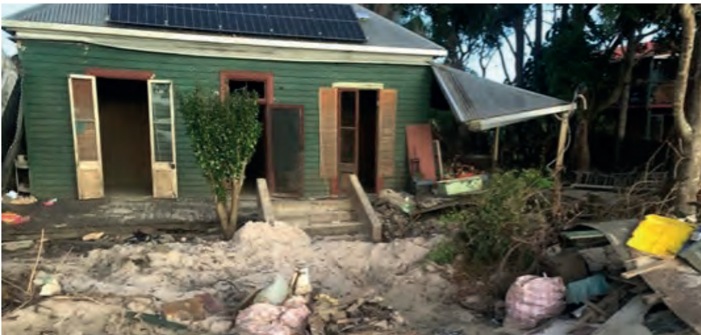
Figure 10: Broadwater residence showing structural damage and large amounts of flood-deposited sand in the front yard. (Photo courtesy of Risk Frontiers 2022)
