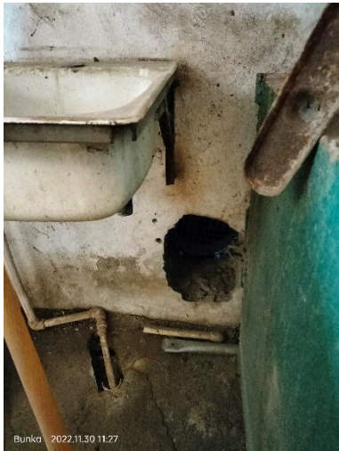
Fig. 22 – Fan heater outlet into staff corridor
