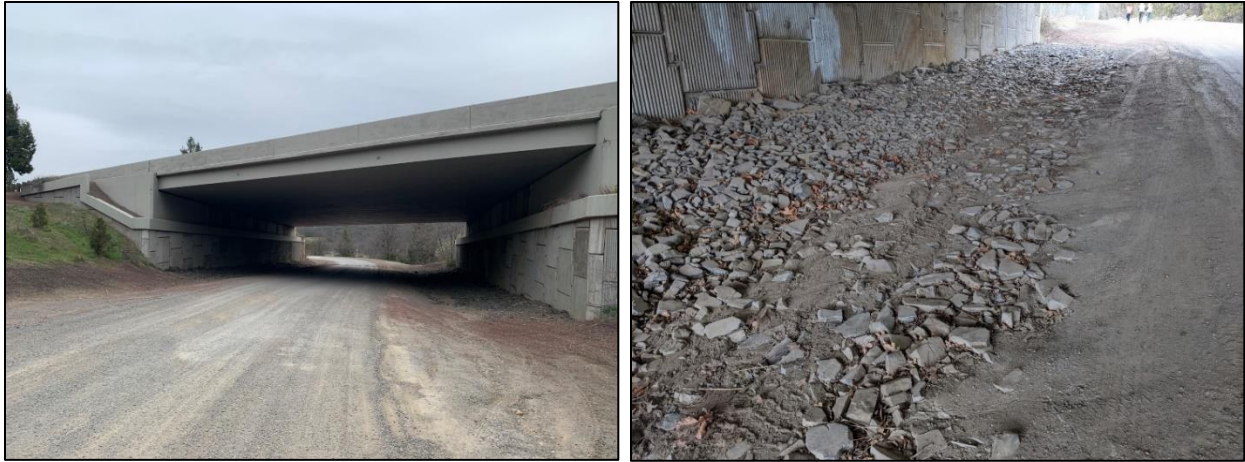
Figure 3-2. Neil Creek Road bridge (left) with I-5 at the top of the image; detail of existing road shoulder materials (right).
