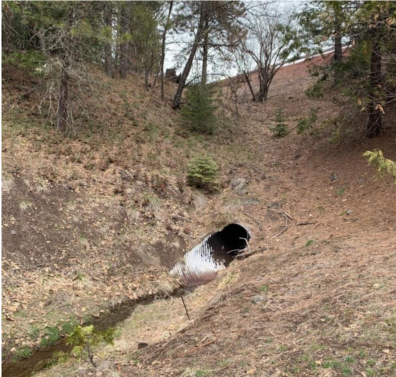
Figure 3-10. Siskiyou Summit culvert inlet with I-5 at the top of the image.
