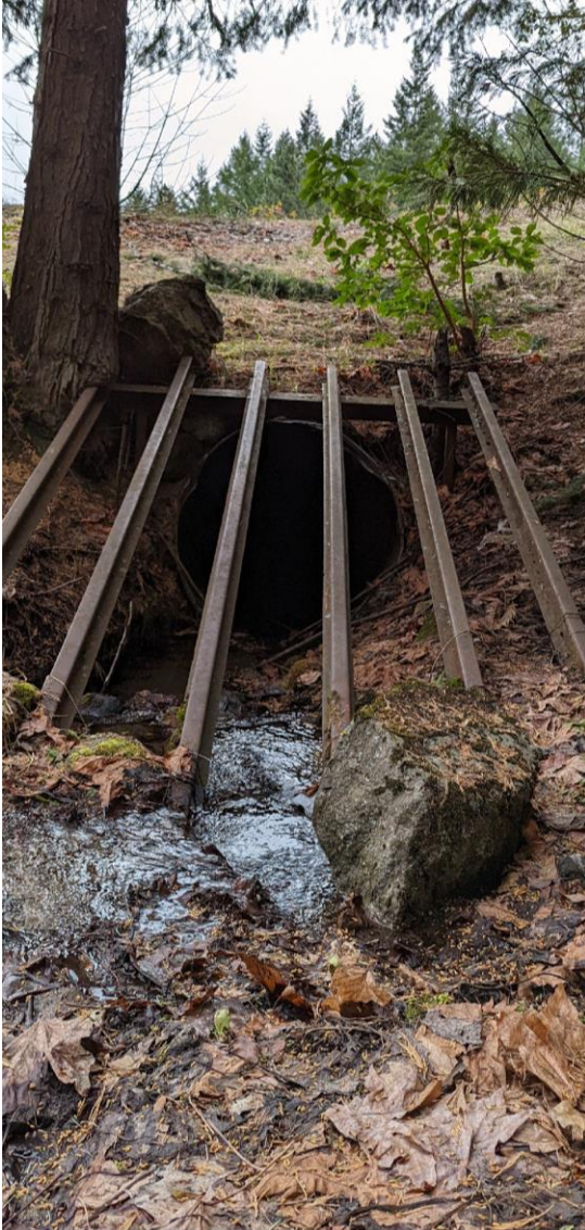
Figure 3-5. Wall Creek culvert inlet with I-5 at the top of the image.
