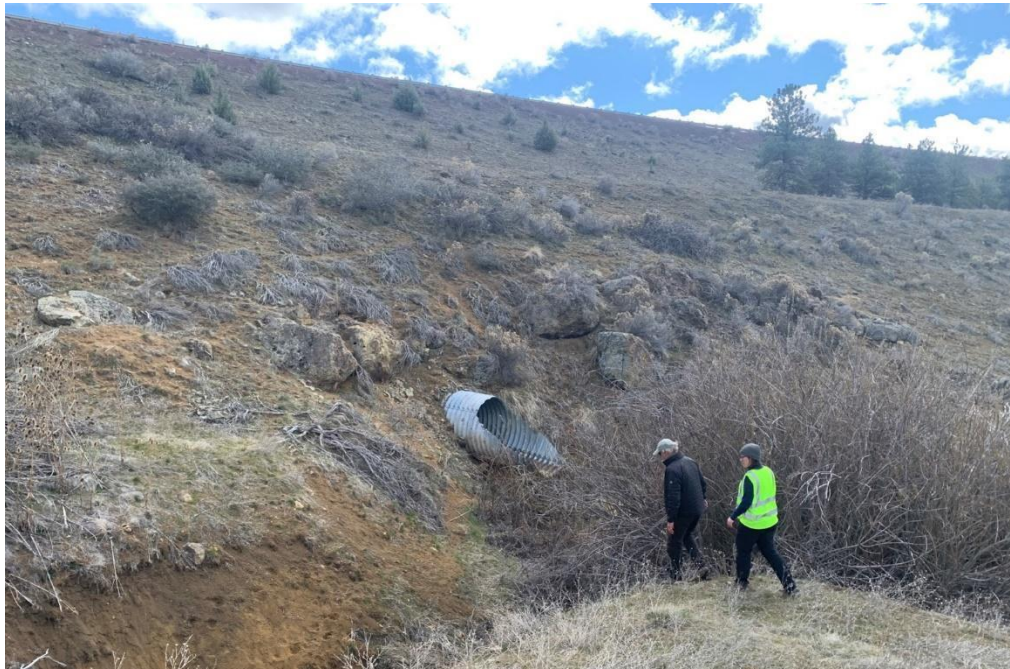
Figure 3-13. Mariposa Preserve culvert outlet with access road bench near the top of the image and I-5 at the top of the image.
