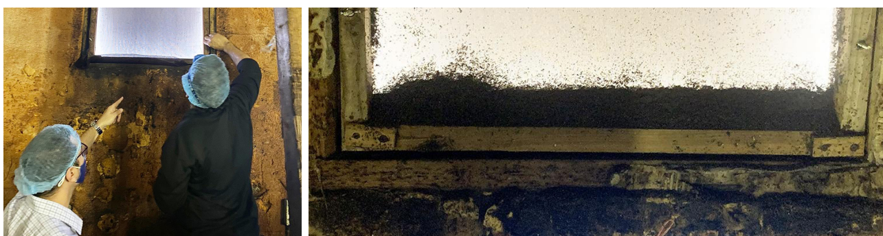
Figure 7. Installing an electrostatic screen treated with biopesticide in a mushroom house, and dead phorids inside the screen.
