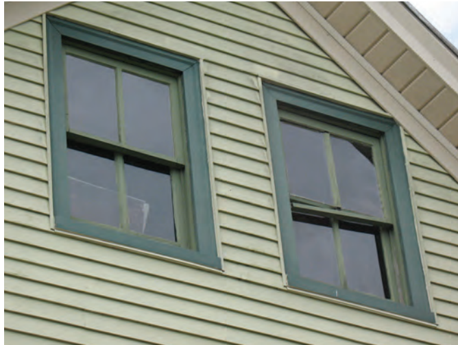
Two-over-two double hung windows are typical of Victorian buildings. This pair exhibits some maintenance problems typical to wood windows which can be repaired.
