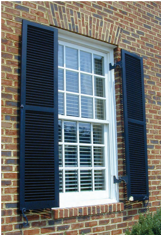
A louvered shutter on a brick building provides a good example of the proper mounting and hardware.
