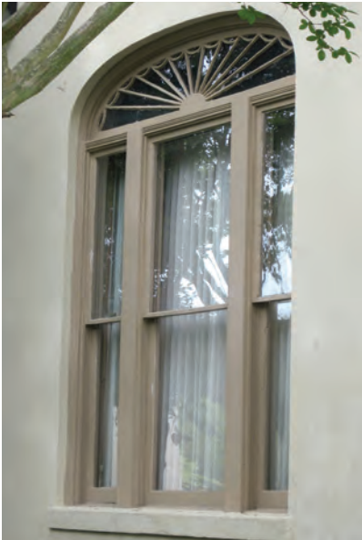
One-over-one double hung windows are common on some building styles. Here, a decorative fanlight transom adds interest.
