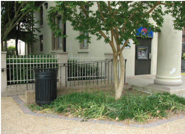
This ramp illustrates sensitive placement and design of handicap accessibility accommodations, allowing access through the side of the porch to the main entrance of the building. All new ramps must meet current building code.
