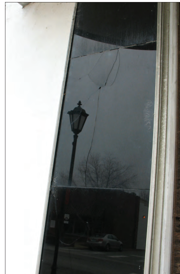
A surviving example of structural pigmented glass on a 1930s facade shows cracks in some of the panels, which can be repaired.
