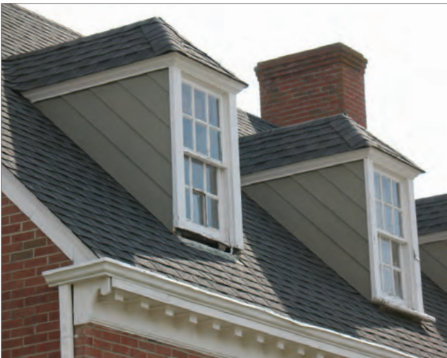
Dormer windows are common on residential form buildings throughout the Main Street area. These dormers have six-over-six divided lights.
