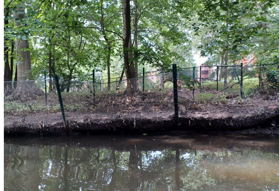
Fences are accumulating sediment and debris, and in places collapsing
