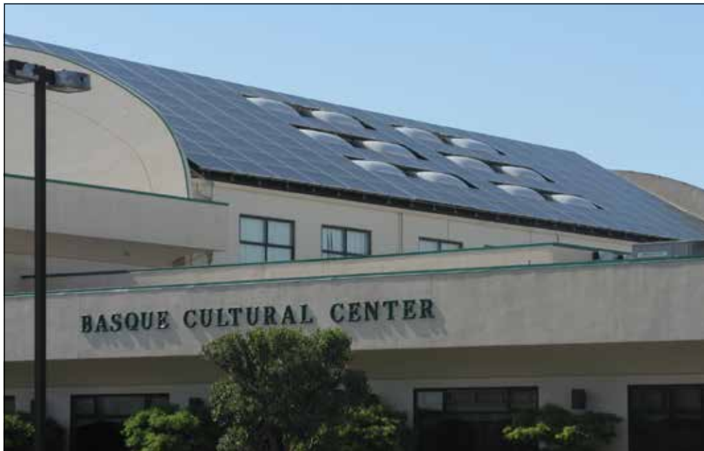
Top: Building and Grounds Chairman, Jean Gorostiague, switched on the solar panels as BCC President (2007-2009) Isabelle Ocafrain Bushman looks on.
