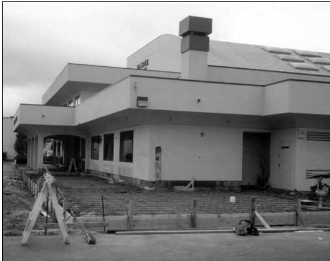
Work on the addition of a Banquet Room and two handicap bathrooms began in 1996.
