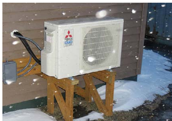
Figure 2. Cold climate heat pump in Alaska
