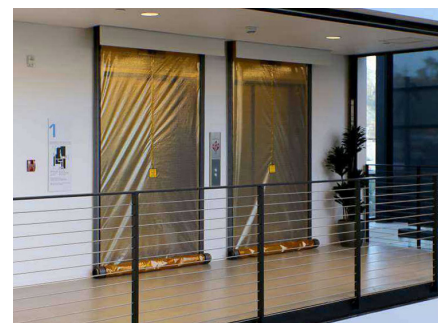
Smoke curtain installed on an elevator. Source: smokeguard.com/gallery
