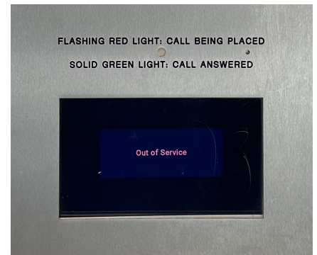
Out-of-service video communication device, on a New York City Subway elevator.
