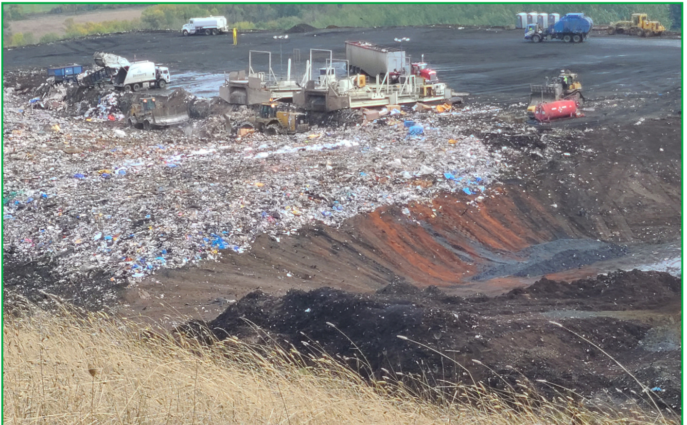
Active working face of Coffin Butte Landfill in Oregon Image Credit: EPA Inspection Report
