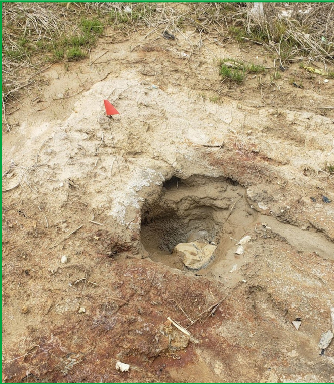
Photo of a SEM exceedance with audible bubbling liquid, Prairie Hill Landfill, Morrison, Illinois Image credit: EPA Inspection Report
