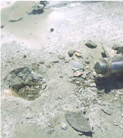
ABOVE: Before application of Surtreat extraction plug crumbles easily.
