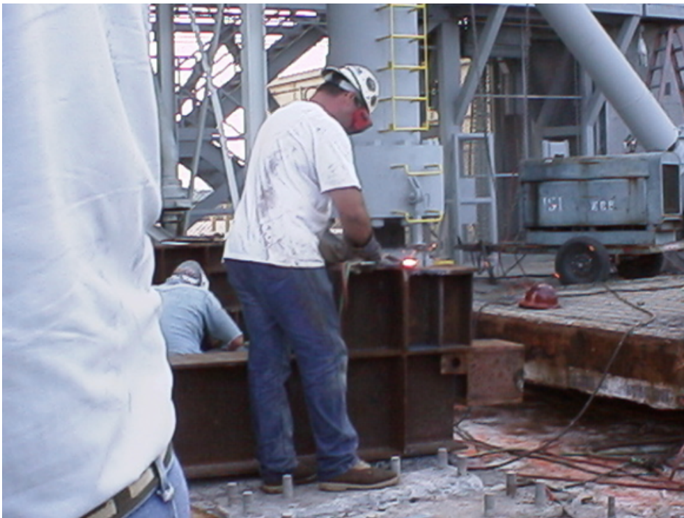
LEFT: Corroded metal elements on the launch pad being repaired and treated to prevent further corrosion to the structure.
