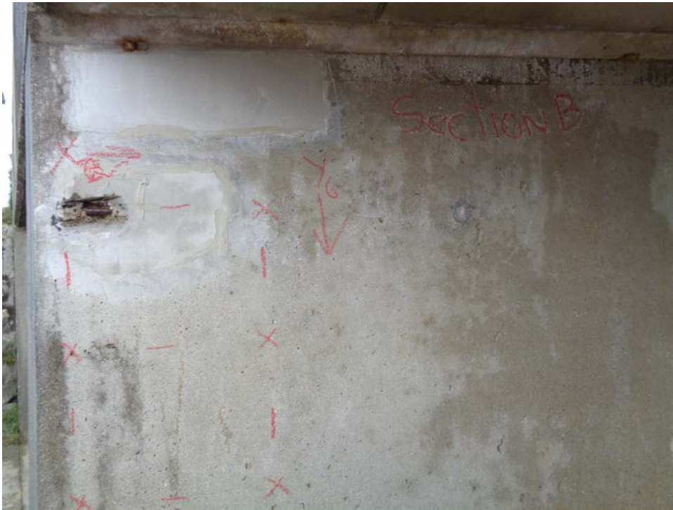
Figure 7 – Sealer still evident after several wettings of the concrete
