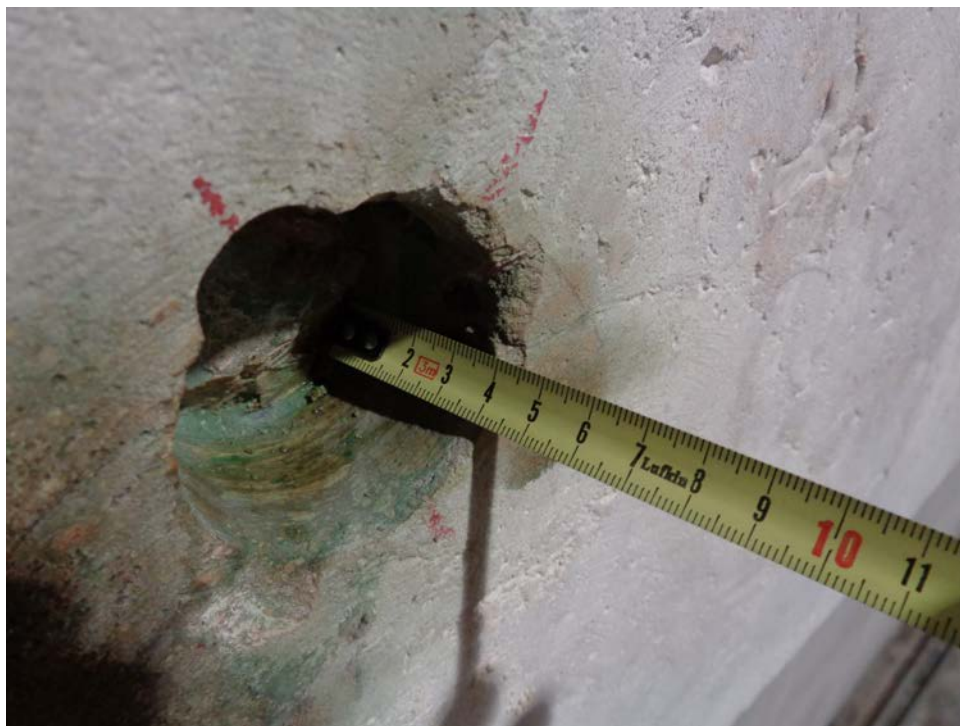
Figure 12 – Core removed over horizontal rebar, and pH indicator applied
