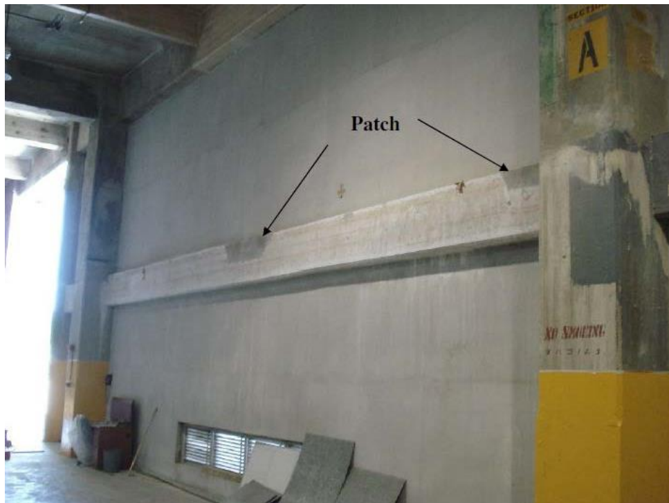
Figure 8 - Section 1 of the ring girder at Building 306 in the Naha Military Port, 2010
