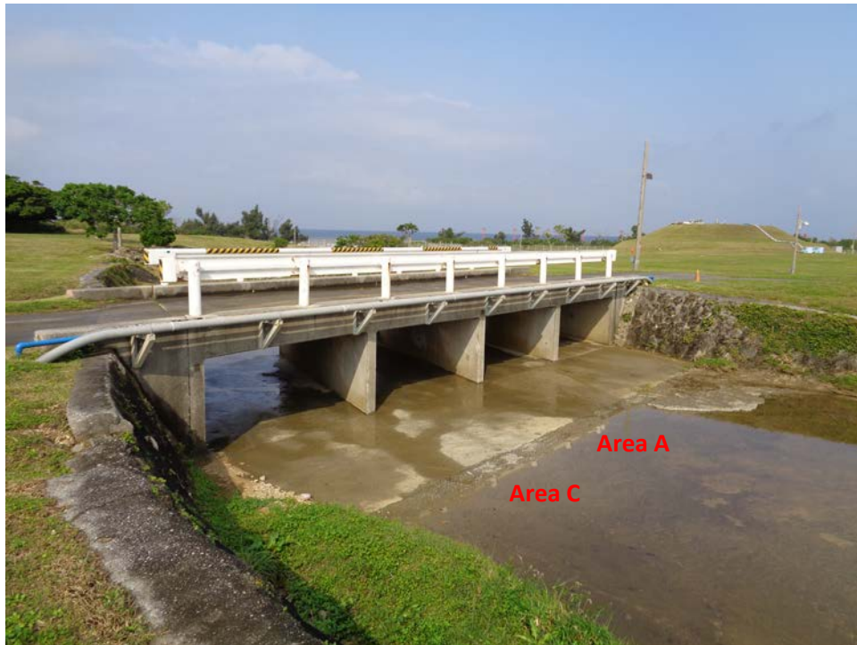
Figure 3 – View from upstream of Bridge 2 at the Kuwae Tank Farm, Kadena AFB, 2016
