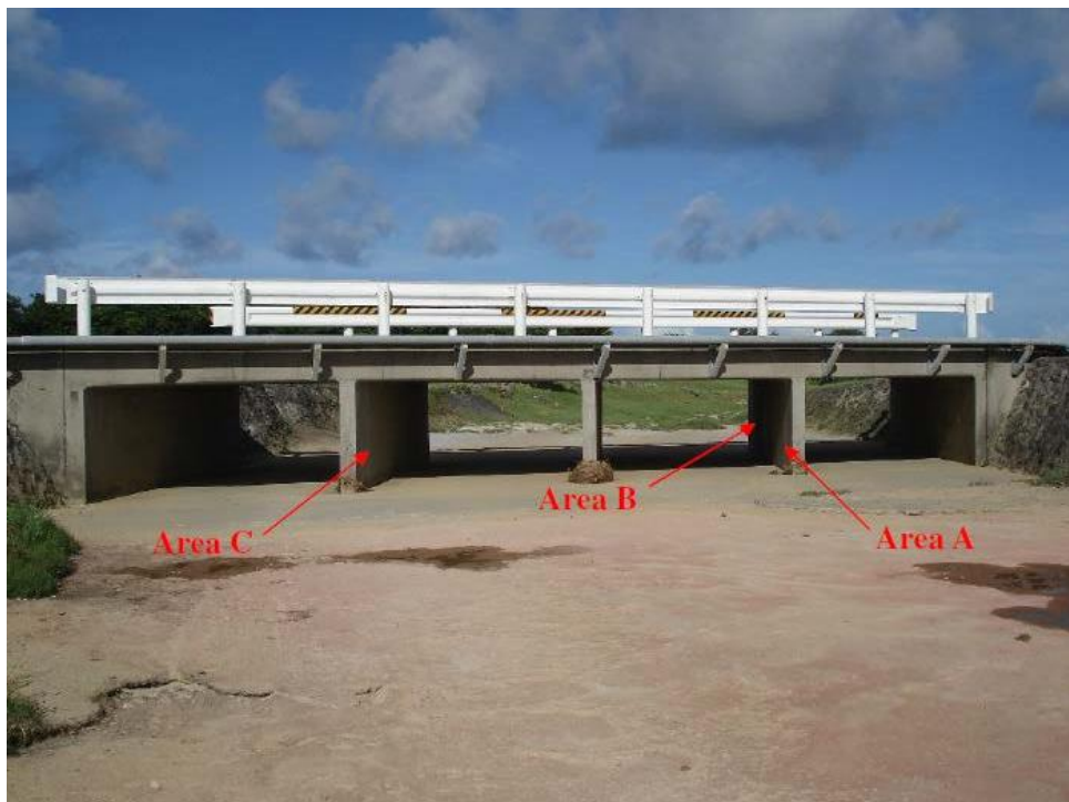
Figure 2 – View from upstream of Bridge 2 at the Kuwae Tank Farm, Kadena AFB, 2010
