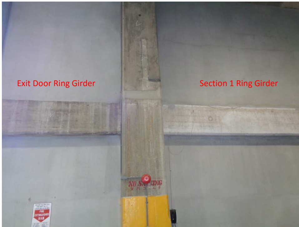
Figure 13 – Visual comparison of section 1 ring girder in to ring girder adjacent to exit door.
