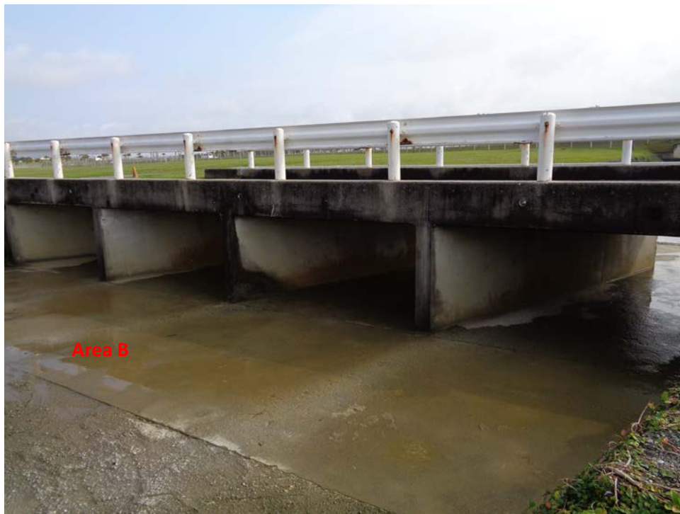
Figure 4 – View from downstream of Bridge 2 at the Kuwae Tank Farm, Kadena AFB, 2016
