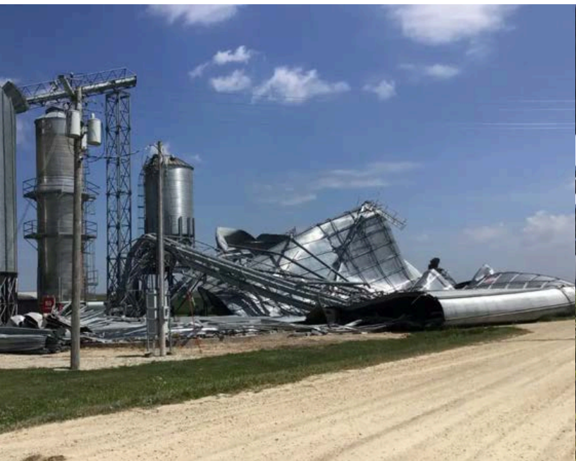
Climate change is increasing incidence of extreme weather events such as the August 2020 Derecho responsible for damage to this farm grain storage. Source: National Weather Service
