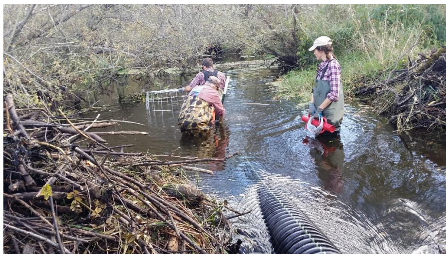
Photo 3. Fence and Pipe flow device installed along Chimacum Creek to address an area with frequent beaver activity.
