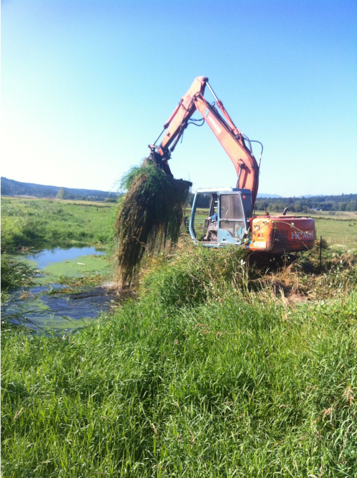
Figure 8. Photo of an excavator with a rake attachment removing canary grass from Chimacum Creek on August 14, 2020.
