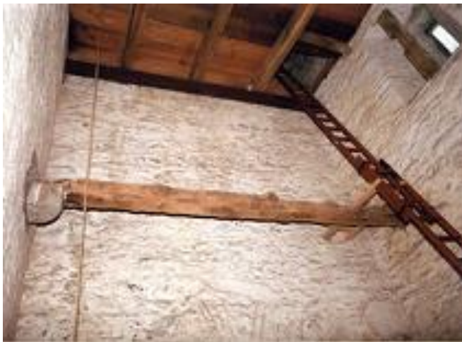
The missing floor in the tower - note the 'forlorn window' on the north face.
