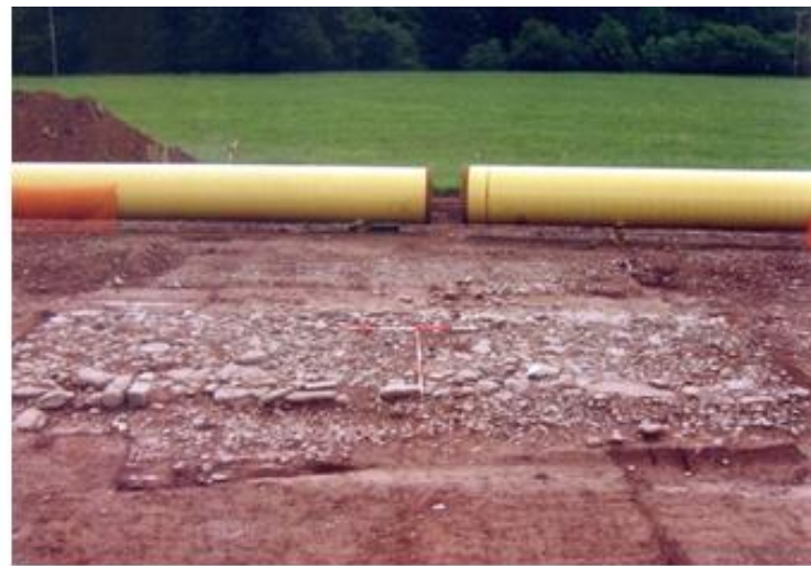
Fig. 3 The road just north-west of Y Gaer crosses from left to right, exposed in 2007 during pipeline excavation. The surface is of packed stone, and the kerbstones can be clearly seen, as can the nearer and further side ditches.
