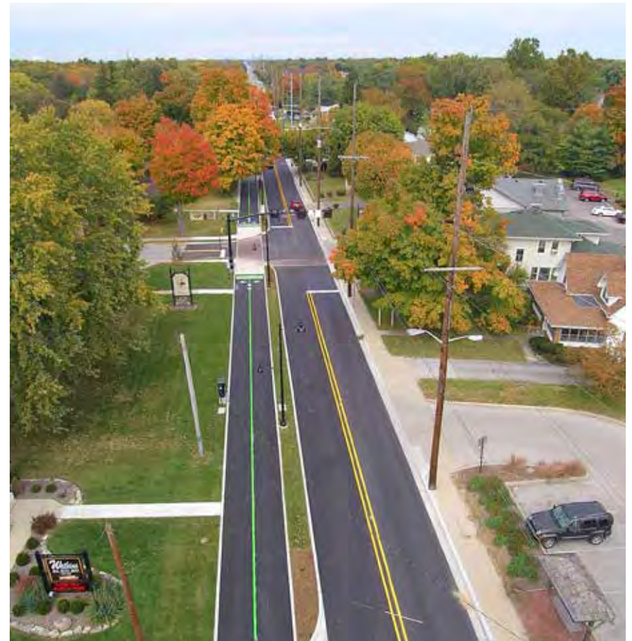
Madison Avenue has been reconstructed in segments to add a multi-use trail, marked crosswalks, and other streetscape improvements.
