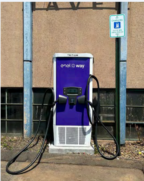
City of New Haven EV Charging Station Source: New Haven Independent
