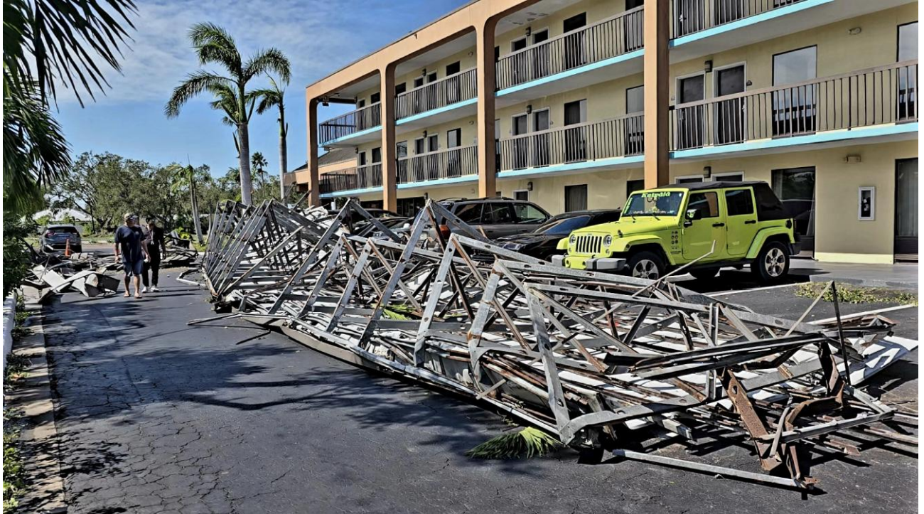
Figure 14: Damage to a Hotel Near Downtown Sarasota
