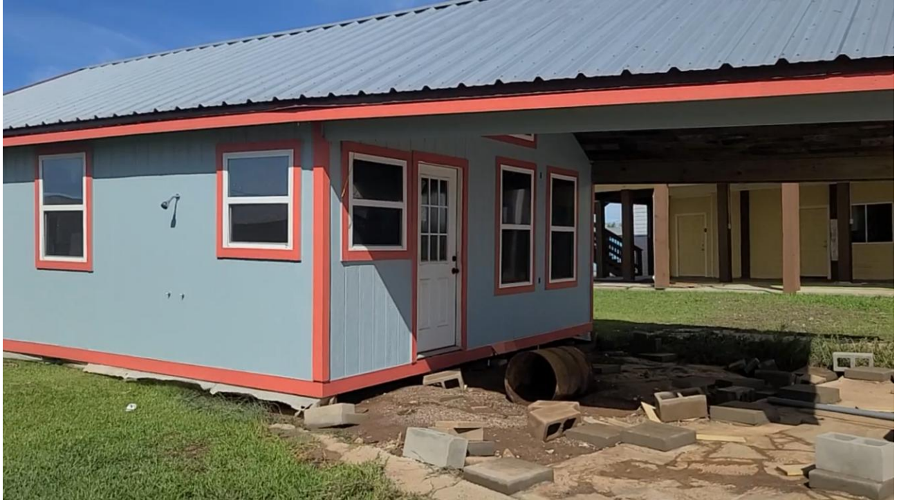
Figure 29: Sargent—Storm Surge Damage
