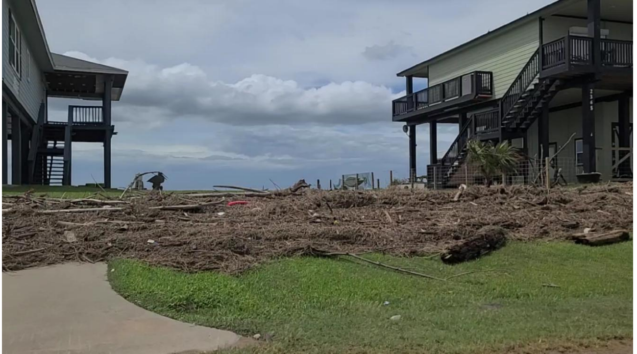
Figure 33: Sargent—Wind & Storm Surge Damage
