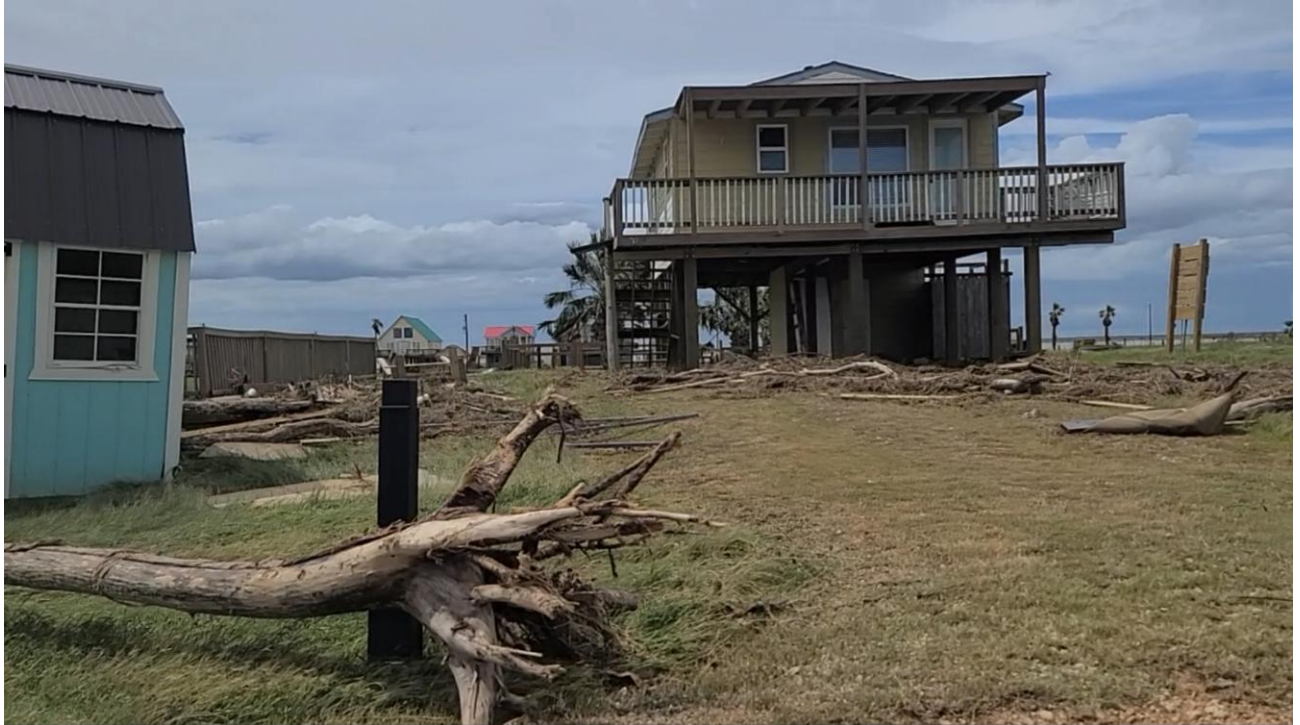
Figure 27: Sargent—Wind & Storm Surge Damage
