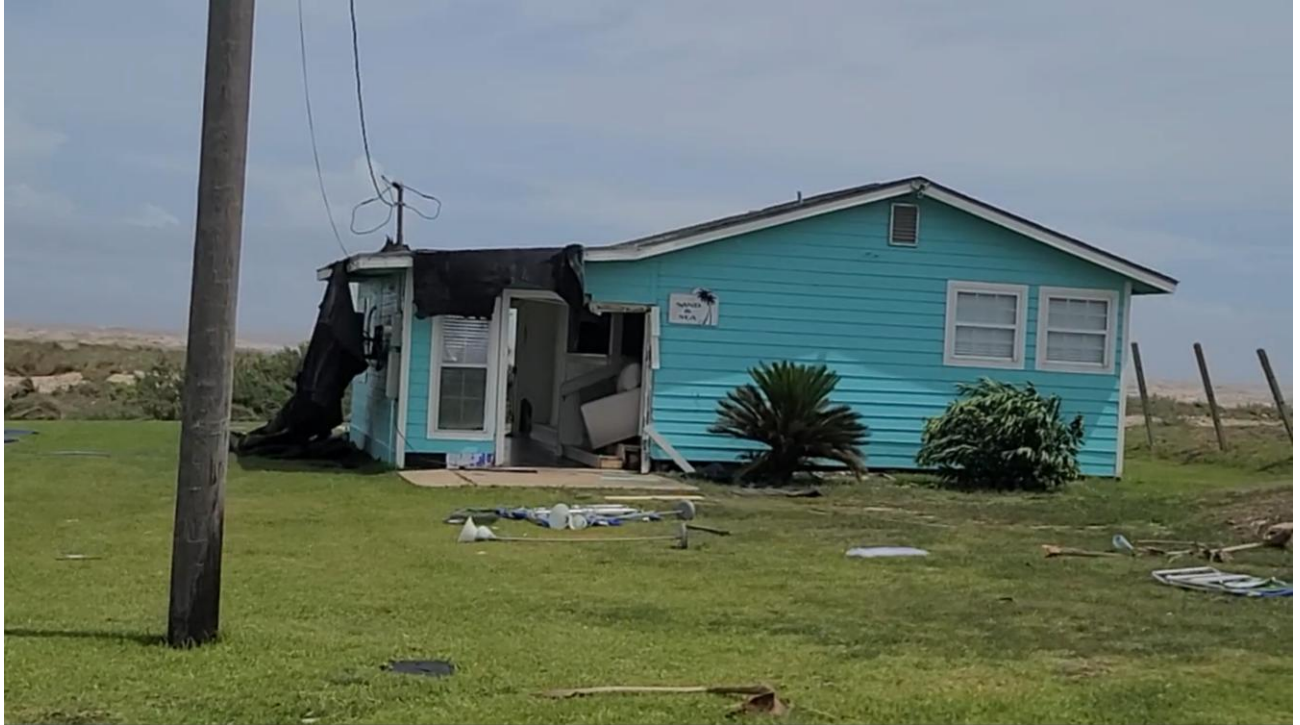
Figure 31: Sargent—Storm Surge Damage
