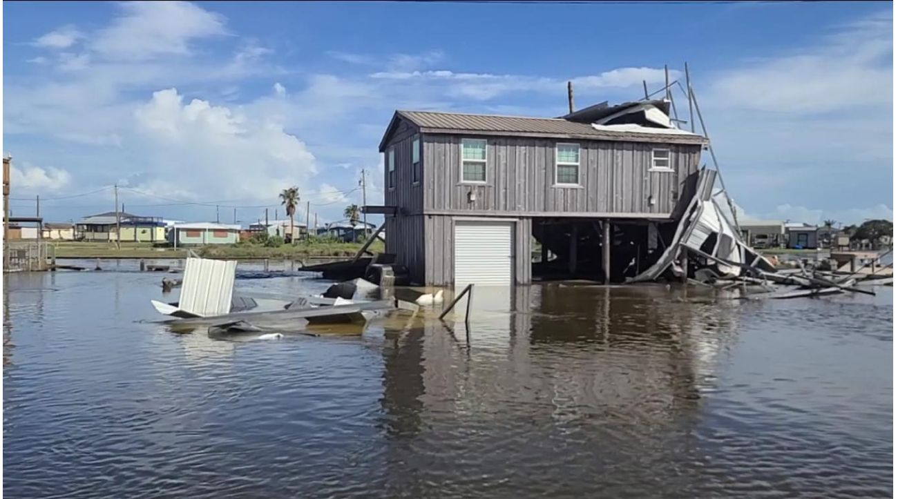
Figure 21: Sargent—Wind & Storm Surge Damage
